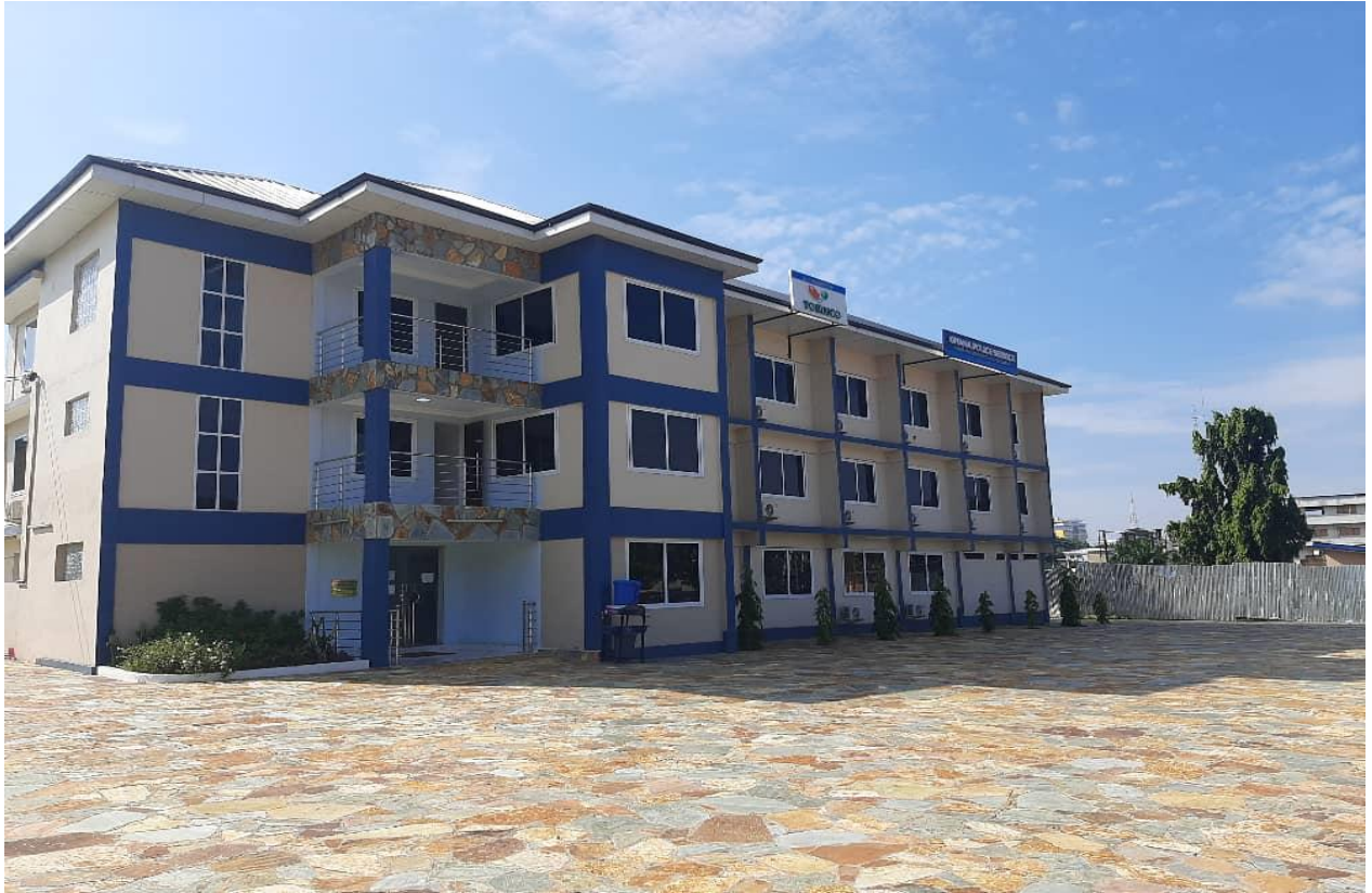
Completed Renovation Work on Senior Police Officers' Residence at The Police Headquarters- Accra
