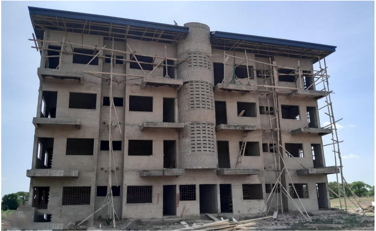
Construction of 4 storey 24 Unit Chamber and Hall Self Contained at Savelugu, Tamale, Northern Region (70% completed)
