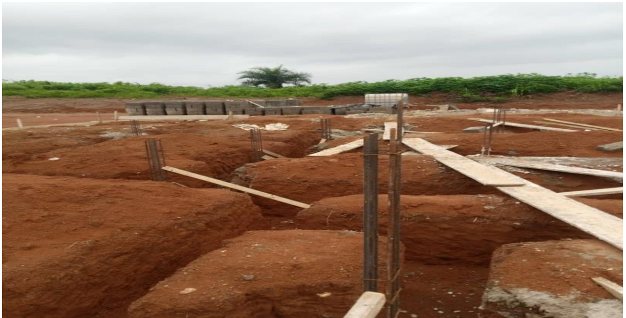
Foundation and footing for the Fire Training College at Bogoso in the Western Region
