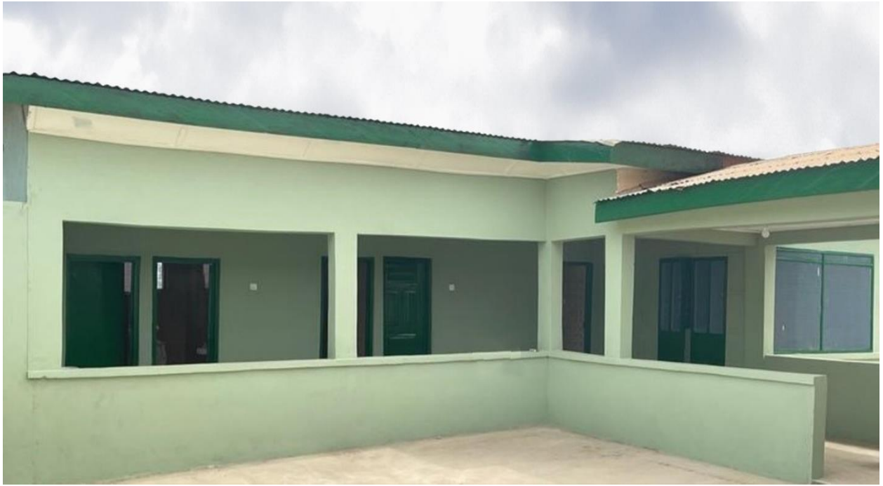
Refurbishment of Instructors' Bungalow at the Ghana Immigration Service Training School, Tapa, Ashanti Region (Compound) (100% completed)
