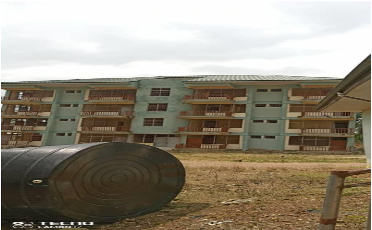
Construction of a 3-Storey, 2-Bedroom Block of 6-Flats, 3-Bedroom Bungalow, and 4-Storey of 24 Flats External Associated Works at Elubo is 85% completed
