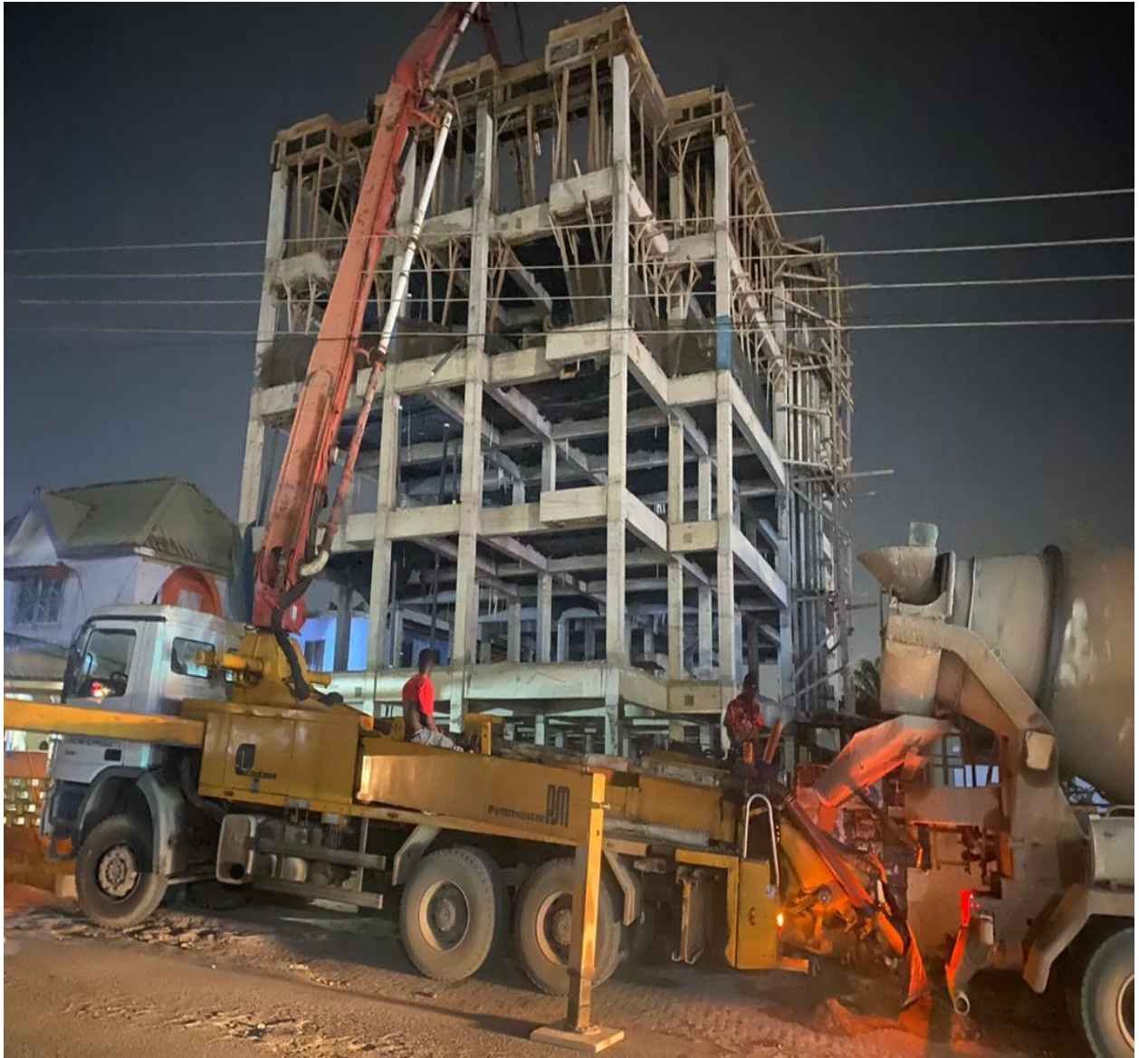
Construction of 4-storey 12 flats comprising 4 Units 2-bedrooms apartments and 8 units chamber and hall apartments at Takoradi Effiakuma, Western Region
