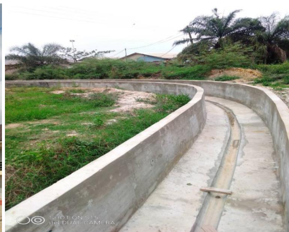
Construction of 1.5m x 1.2m Reinforced Concrete Storm Water) at Sefwi Dwenase Market at Sefwi Wiawso MA
