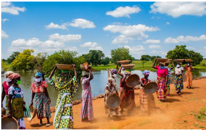
LIPW Beneficiaries at Work On A Small Earth Dam At Kulsaboug In Nabdram District
