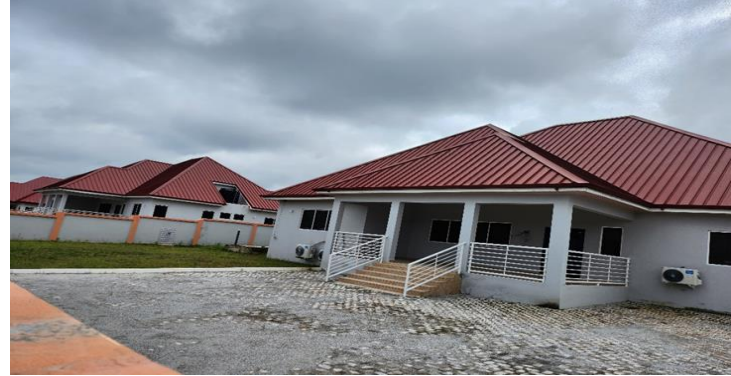
CONSTRUCTION OF 3NO SENIOR STAFF BUNGALOWS FOR REGIONAL COORD COUNCIL AT SEFWI WIAWSO
