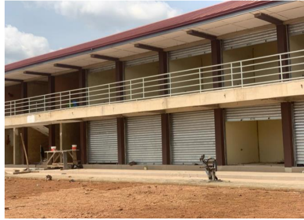
Construction of 40 Units 2-Storey Lockable Stores at Salaga Market at East Gonja
