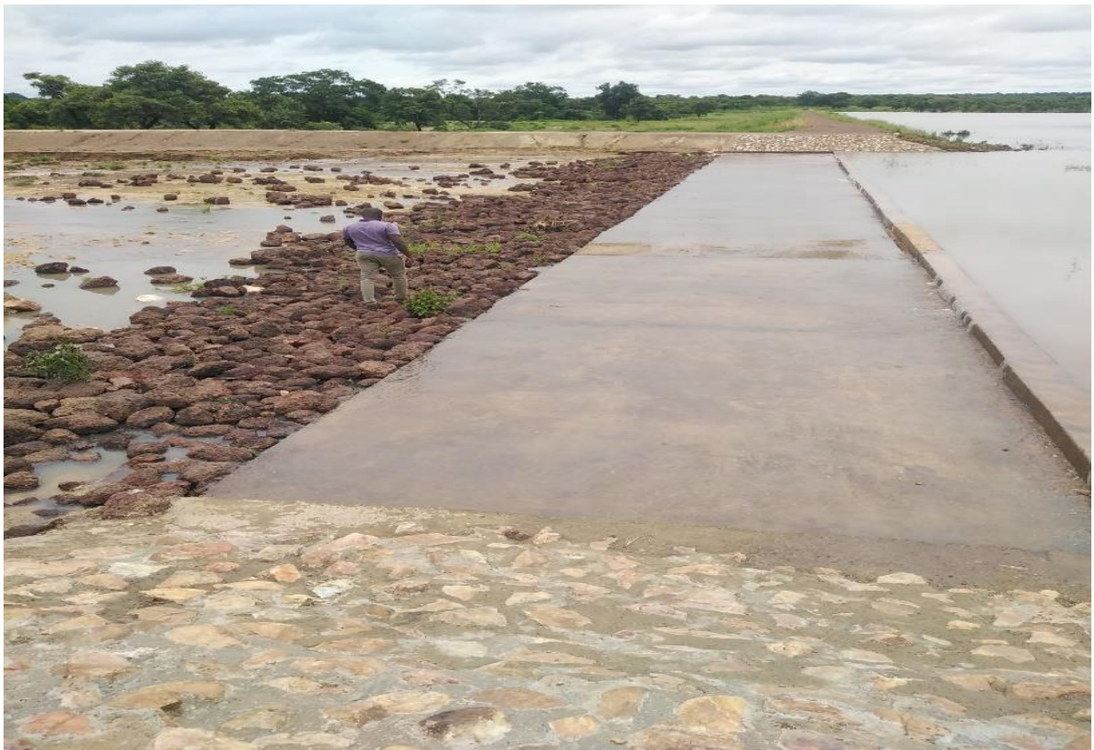
Spilling of completed Small Earth Dam at Kataa in the Upper West Region
