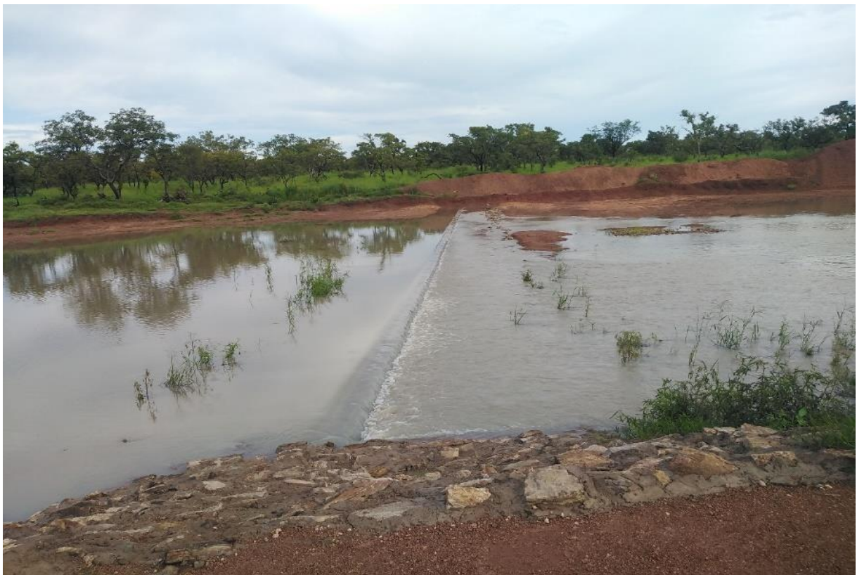
Spilling of completed Small Earth Dam at Duong in the Upper West Region
