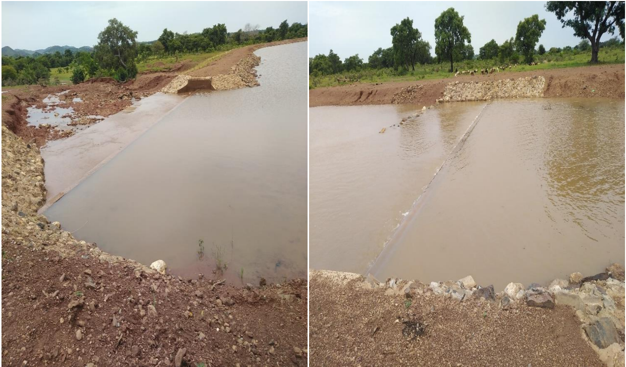
Spillways of Small Earth Dam at Namolgu in the Upper East Region
