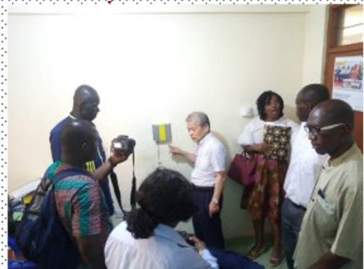
EQ guard installed at Weiija-Gbawe Municipal Assembly for the detection of earthquake early signal and issuance of alarm.
