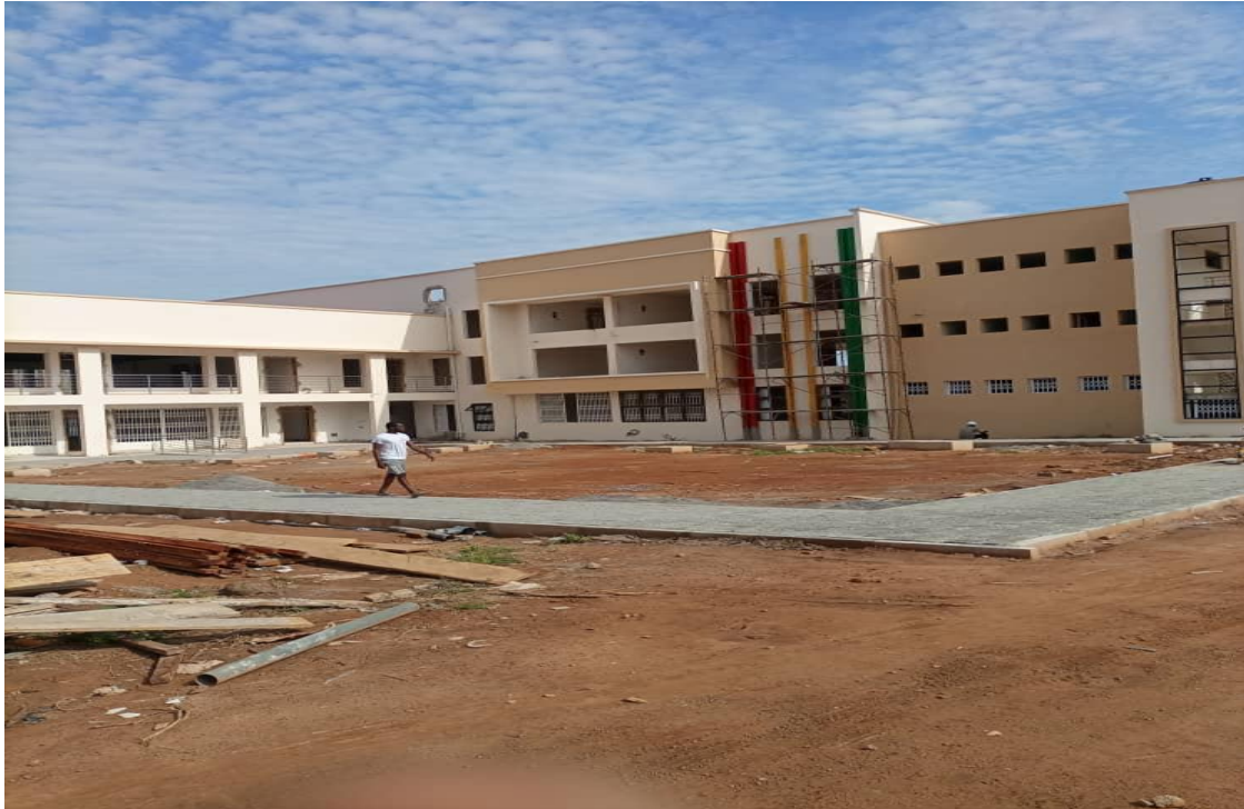
ON-GOING 1NO. 3-STOREY ADMINISTRATION BLOCK FOR SAVANNAH REGIONAL CO-ORDINATING COUNCIL (RCC) AT AMONGO
