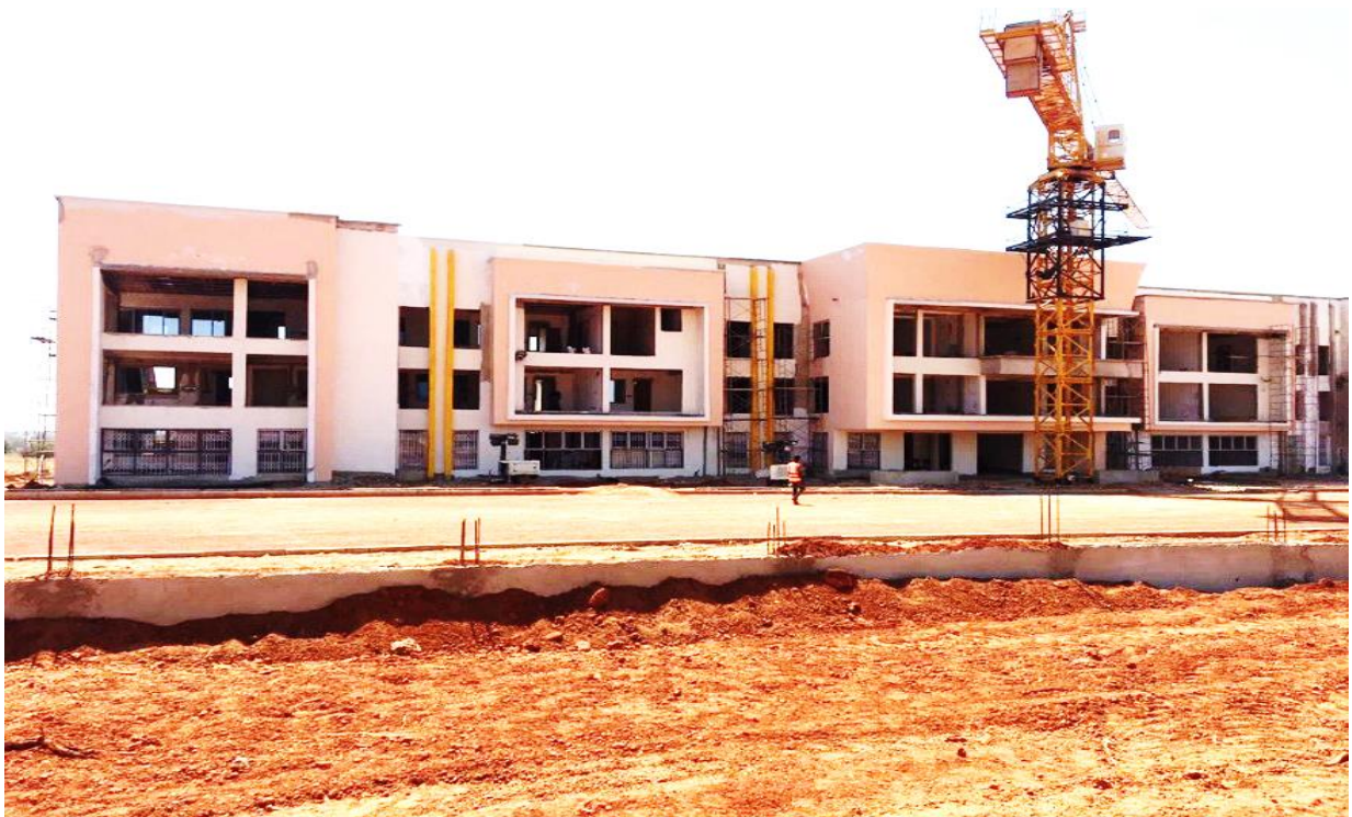
ON-GOING 1NO. 3-STOREY ADMINISTRATION BLOCK FOR NORTH EAST REGIONAL CO-ORDINATING COUNCIL (RCC) AT NALERIGU
