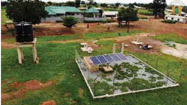
COMMUNITY WATER SYSTEM, BREFOR NAPAARE, LAWRA, UPPER WEST
