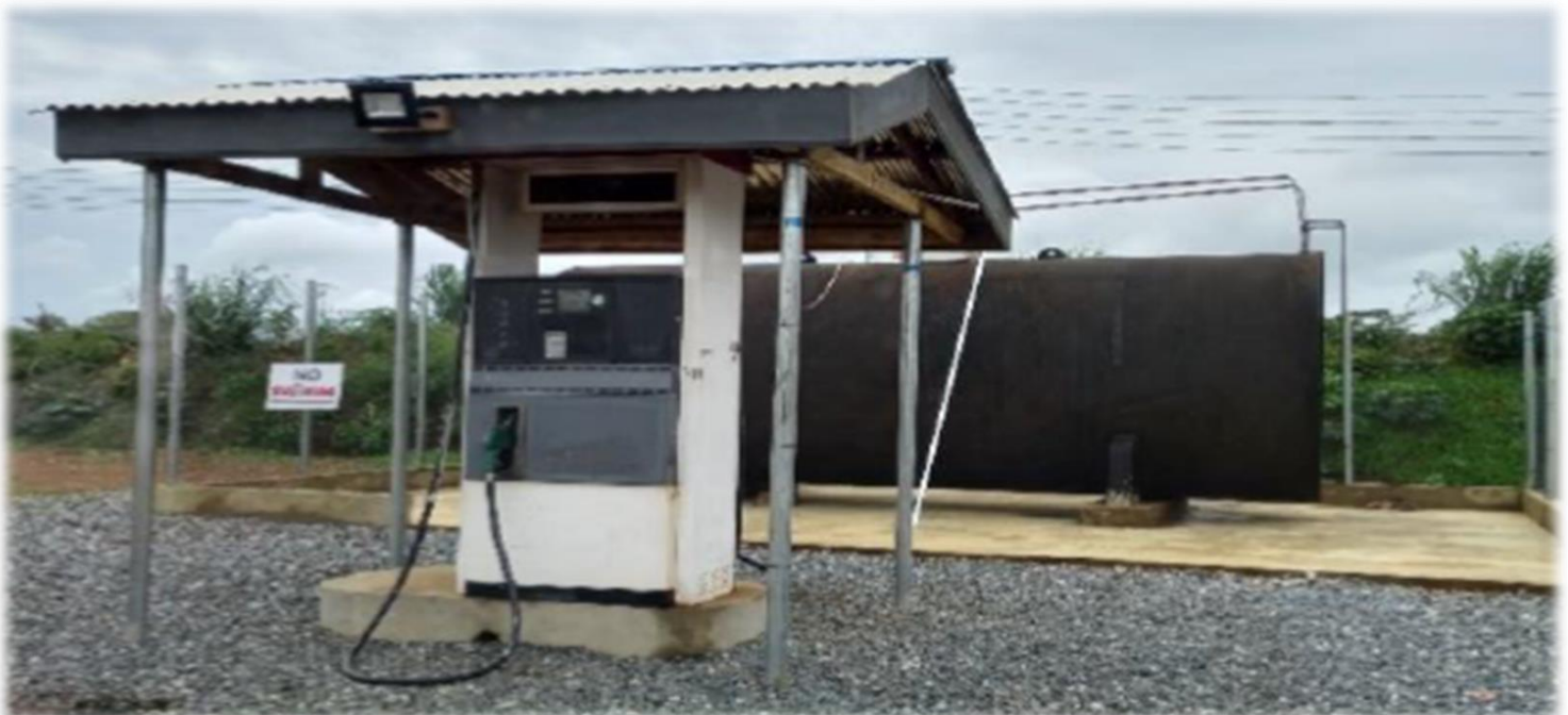
Fuel Station at Vuluxx Yard
