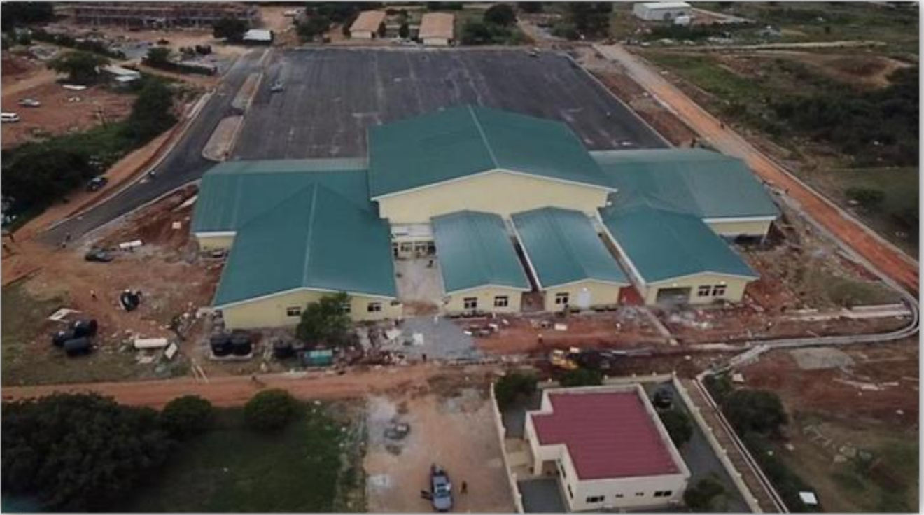
Aerial View of Completed Officer Cadet's Mess at the Military Academy Training School (MATS), Teshie under the USD100M Military Housing Project
