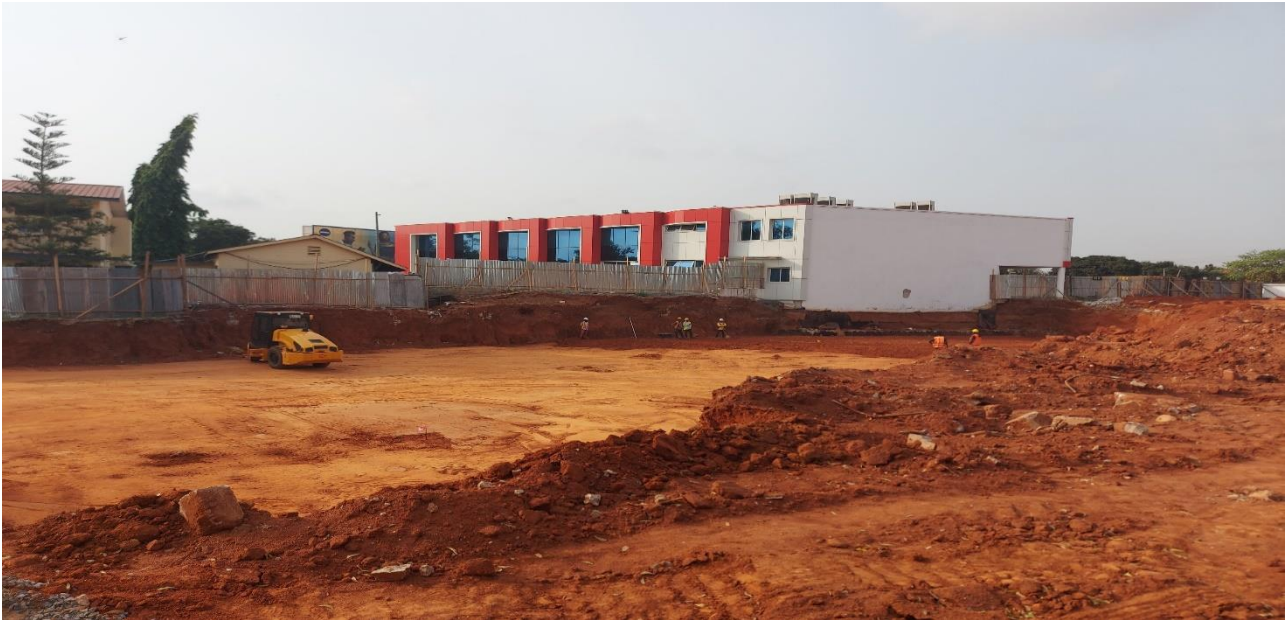
Construction of Lands Commission Head Office Building Construction of GARO Phase II
