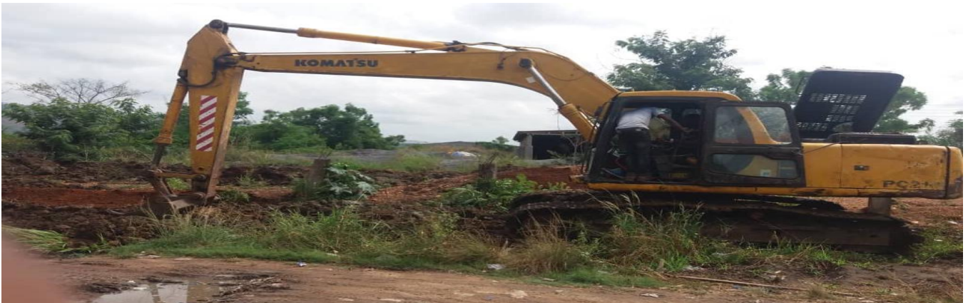
Creation of channel to pave way for free flow of water at Adumanya in the Shai Osu-Doku District
