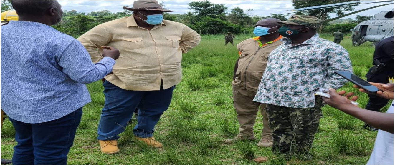
Clearing of debris in the building collapse at Akyem Batabi in the Asin Manso-Akroso District.
