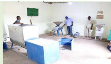
Multi-purpose Processing equipment installed
