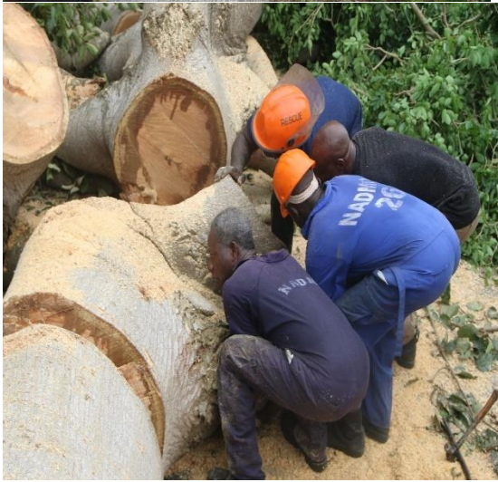
NADMO and GNFS strenuously clearing a road of hazardous trees that fell across it and also on live electrical cables in a residential area near Achimota School
