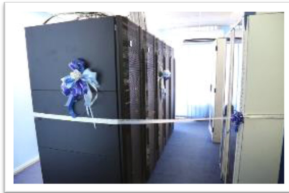
Very Small Aperture Terminal (VSAT)
