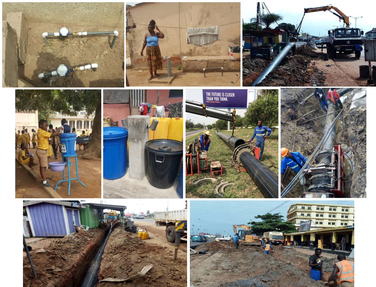
Water projects in Low income communities under the GAMA water and Sanitation Projects
