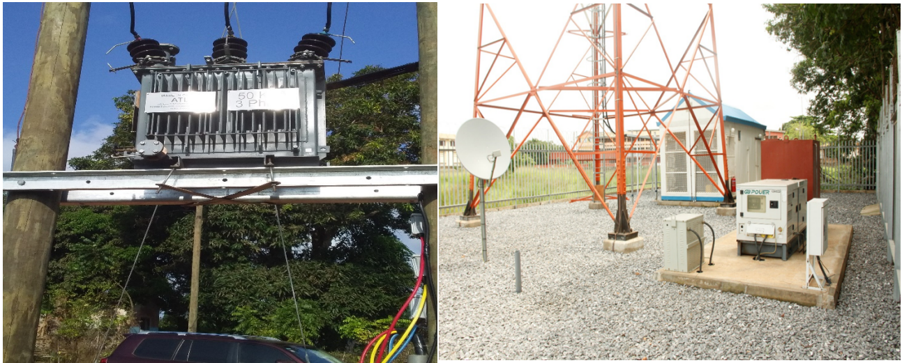
DTT transmission site
