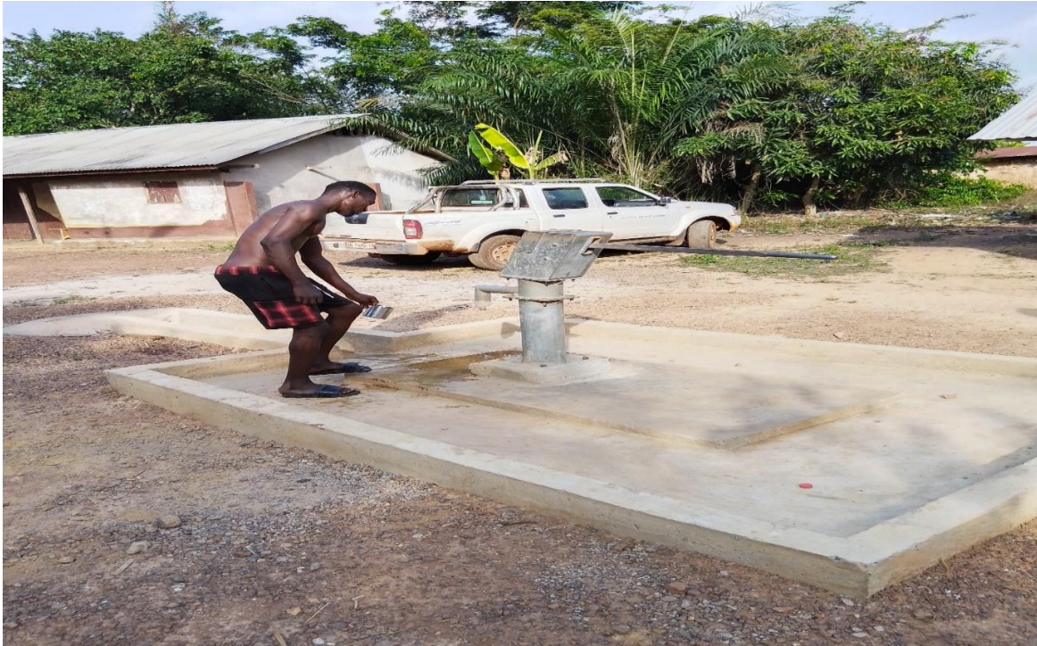
Drilled Borehole fitted with Pump at Sonka
