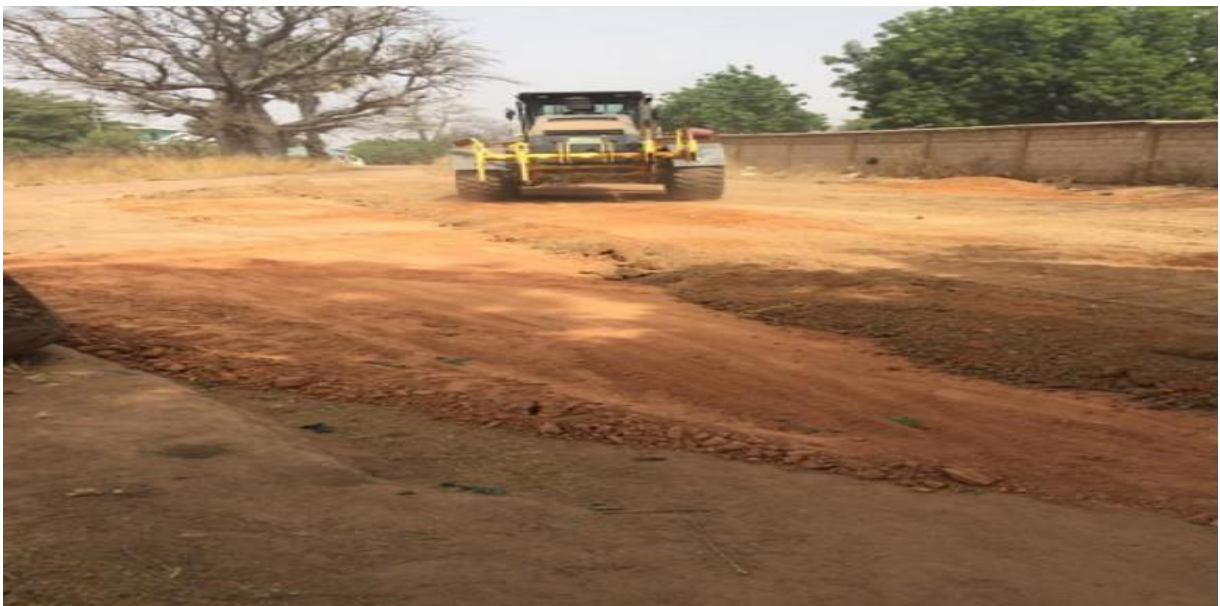
Reshaping and spot improvement of 10km of roads in Dachio, Zonno-Zori and Kumbosigo
