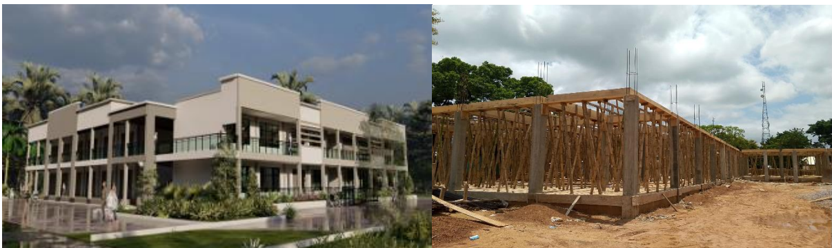
Artistic impression and Actual work done on the construction of 1. No 2 storey shopping centre
