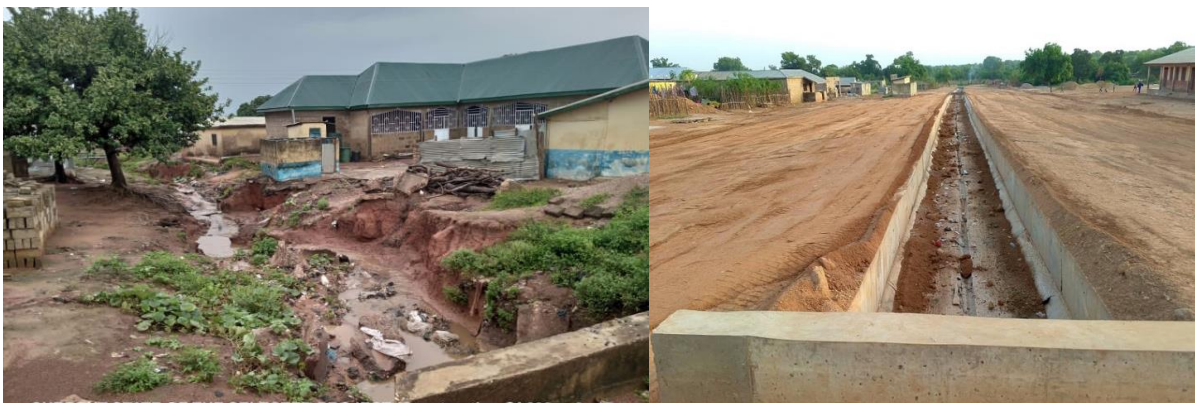
Before and After the construction of the storm drain from Ngaripe to Al marana
