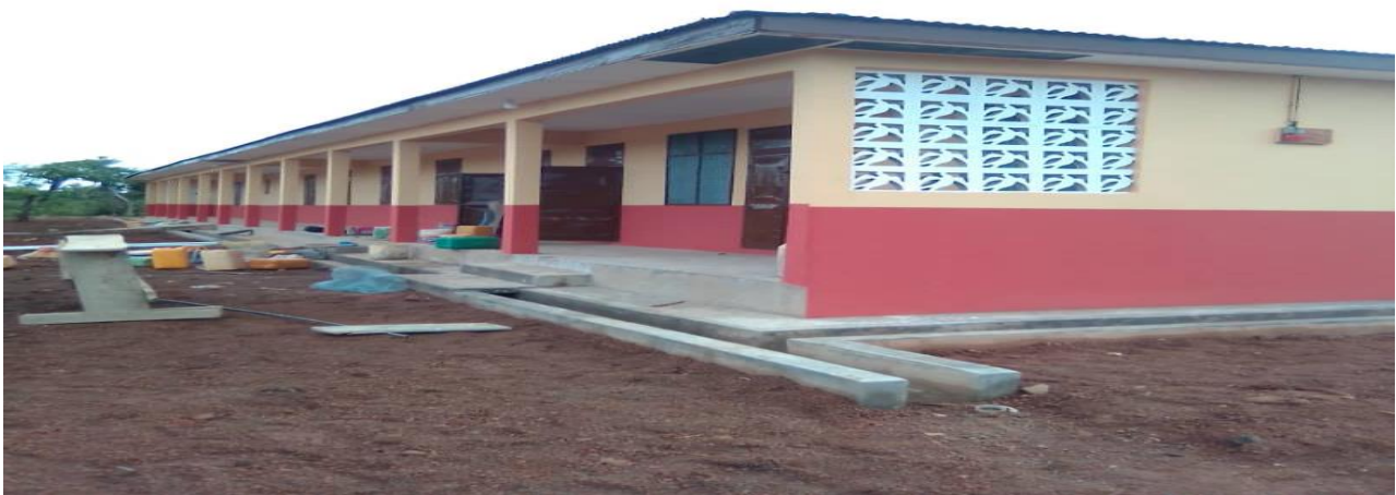
Constructed 3No. 3-unit classroom block with ancillaries at Kalidu, Bombontey and Ntereso
