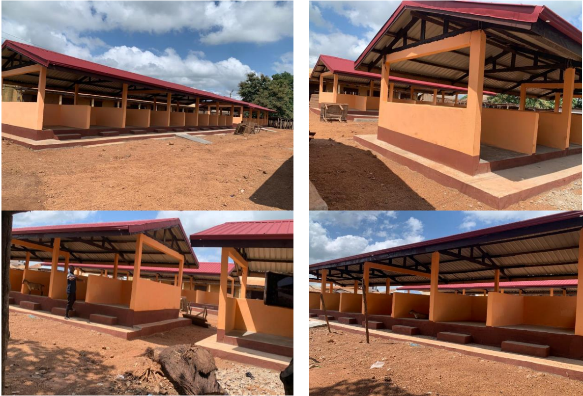
Figure 8: Rehabilitated of 2No. 20-Unit and 2No. 14-Units Open Market Stalls at Chamba Market
