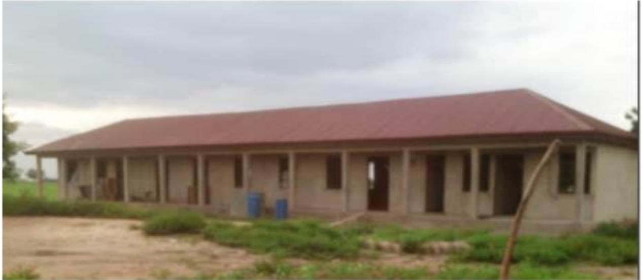
CONSTRUCTION OF 1NO.3UNIT CLASSROOM BLOCK, 4 SEATER KVIP TOILET, CHANGING ROOM AND 2UNIT URINAL AT DIKPUNG
