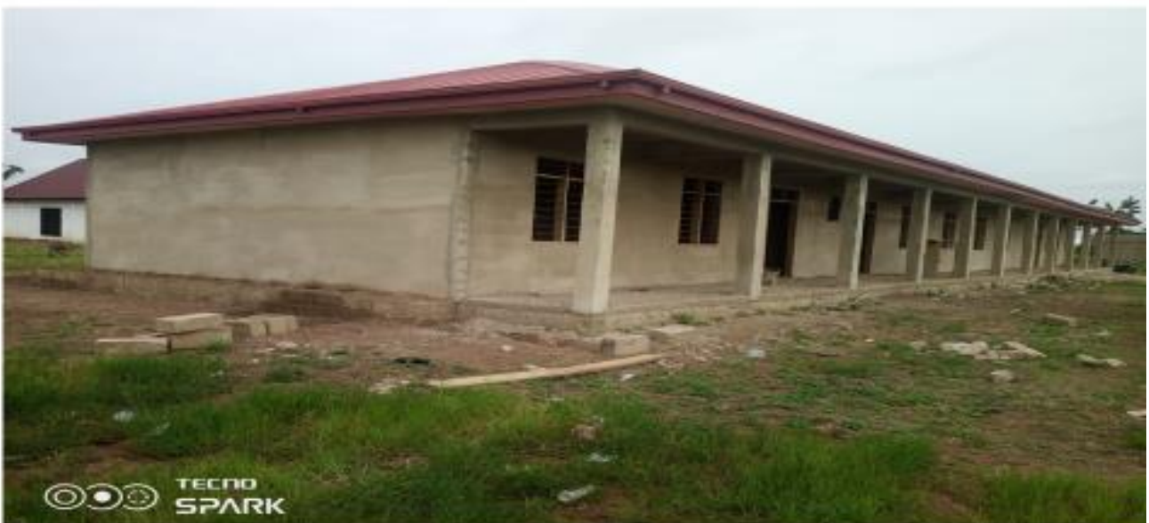
CONSTRUCT 1 NO.3 UNIT CLASSROOM BLOCK, 4 SEATER KVIP TOILET, CHANGING ROOM AND 2UNIT URINAL AT KATANI
