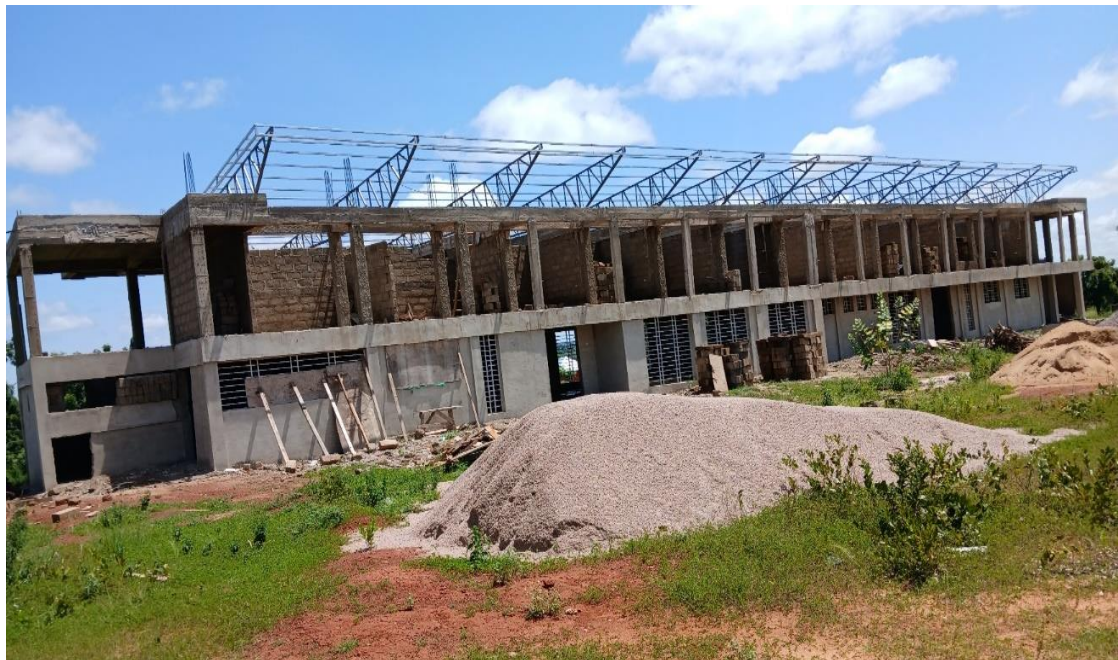
Complete Construction of 2-storey Commercial Building, drain and Paving Works at Nalerigu
