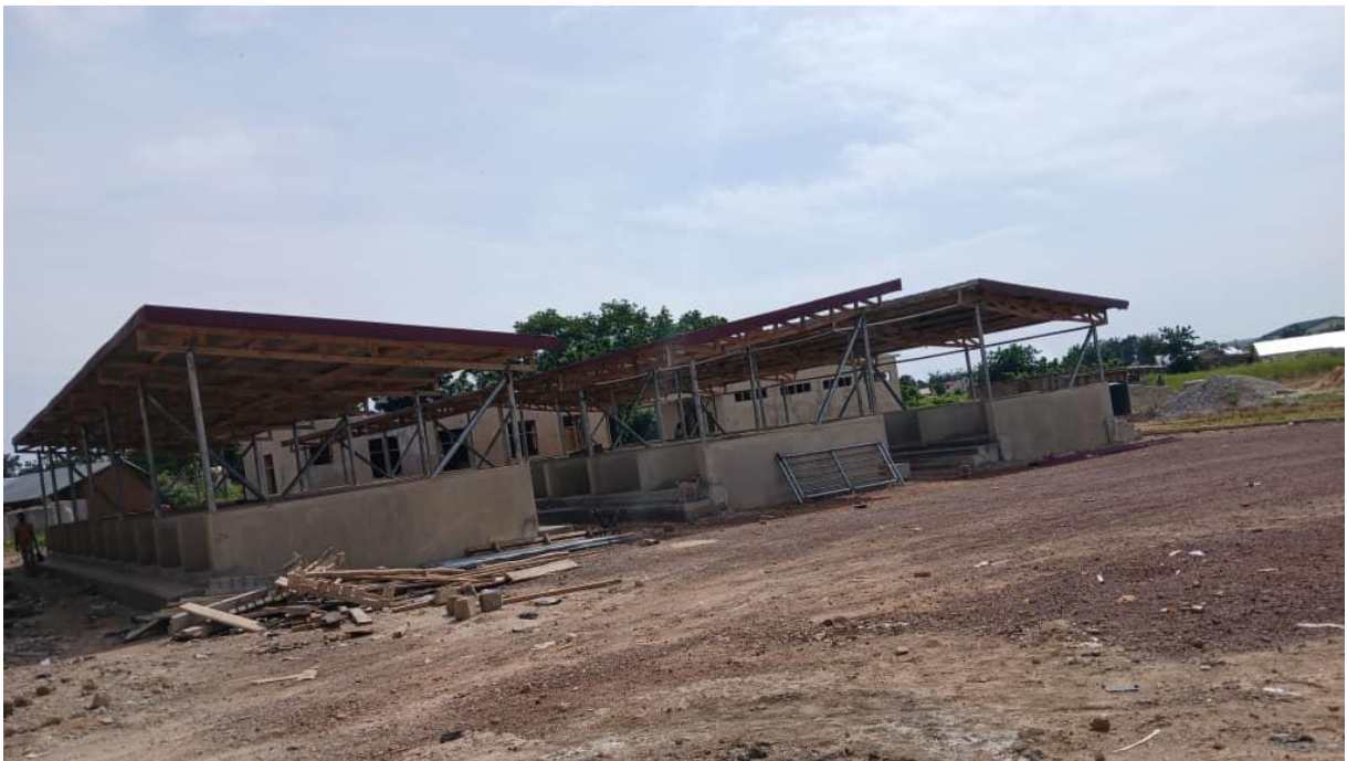
Construct 75NO. Stalls, external works, washrooms, butchery, paving of walkways, cars and lorry park at Gambaga
