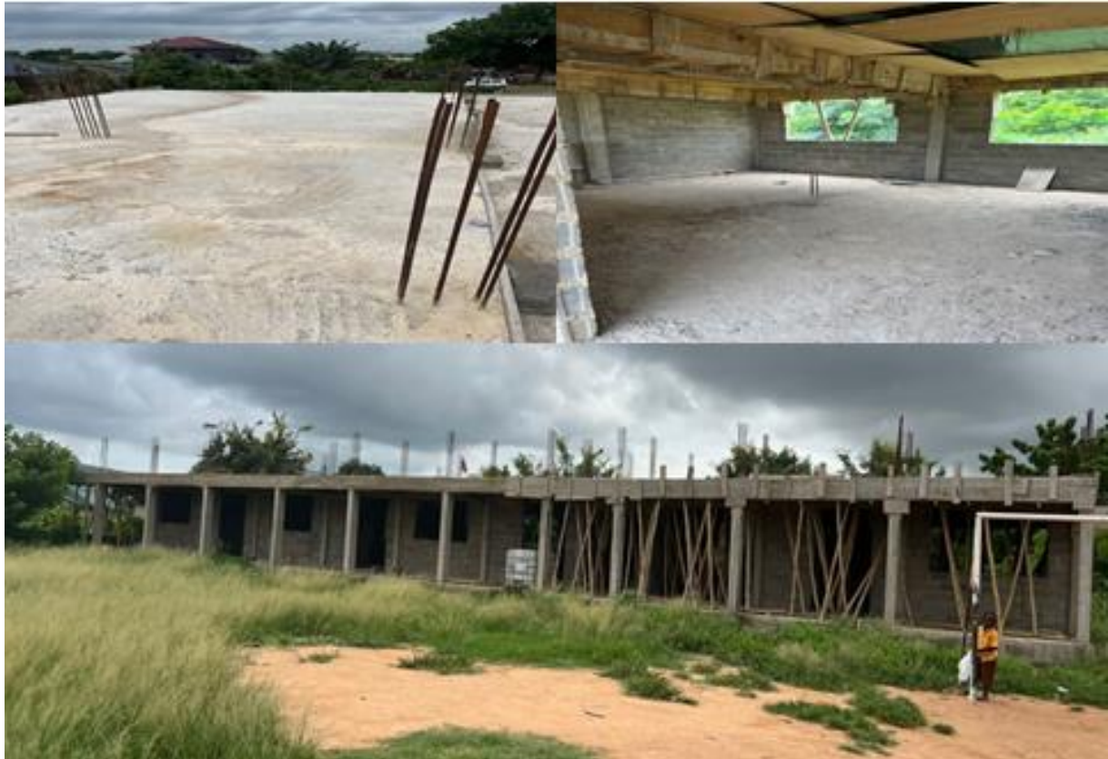
Constructed 1No. 2-Storey 6 Unit Classroom Block With Ancillary Facilities at Nganoman (Block Work Completed)
