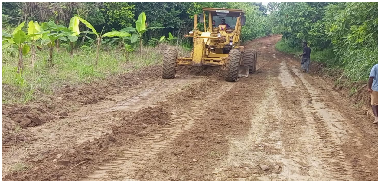
Reshaped 20 km Feeder Roads (Kwahyia to Koramameng to Akorabo, Roman Junction to Gariba Zongo, Ministries to Jehovah Rapha, SDA road, Dr Mabel to Pinto, Wedokum road and Dan Villa
