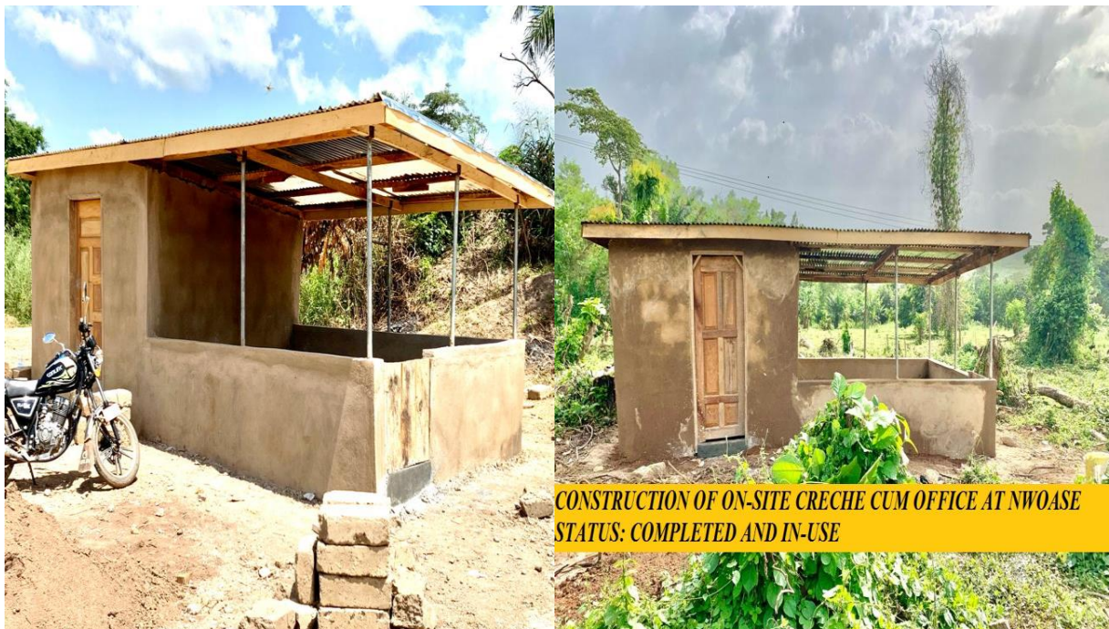
Figure 4: Constructed 4No. Creche, office and 4No. Temporary On-site toilet at Nkonsia, Ayayo, Nwoase and Branam
