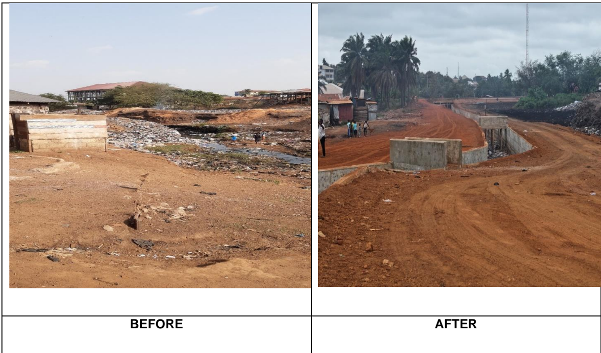
Constructed a Reinforced Concrete Storm Drain (500 x 3x 2.5) of 0.9M U-Drain and Levelling to Reclaim 3 Acre old Dump site
