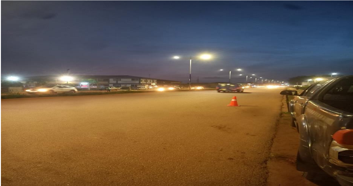
Installed 60No double armed streetlights (2.7km) and 4No, Traffic signals (Penkwasi traffic light to New Dormaa)
