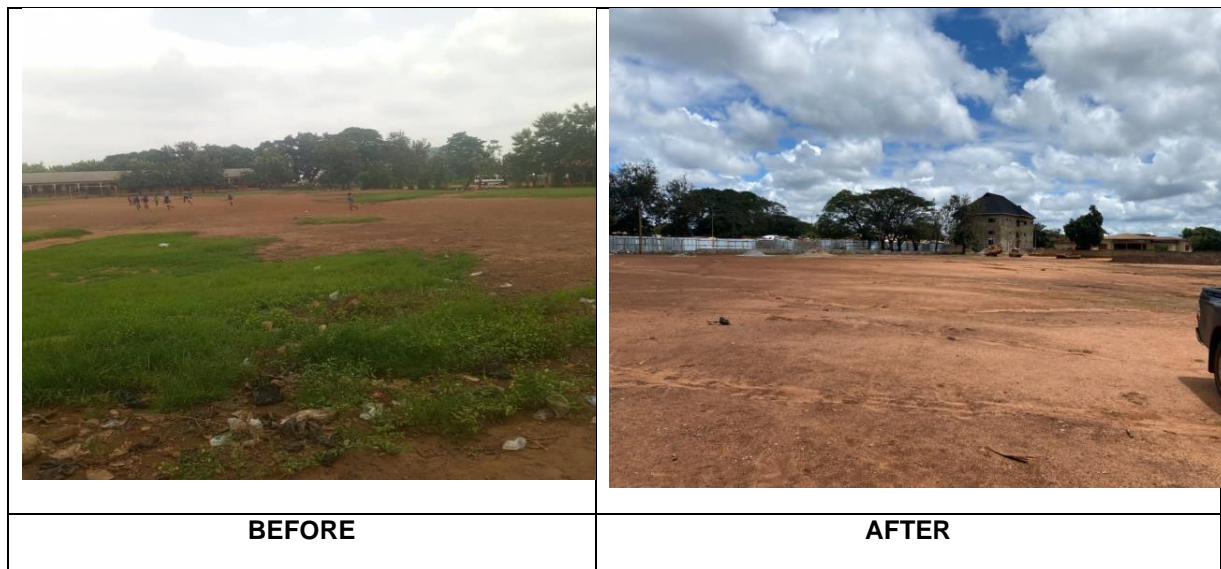
Construction of 1No football Court, volley, Tennis Court area Electrical Supply lighting system, change Room and sanitary facilities (Abesim)
