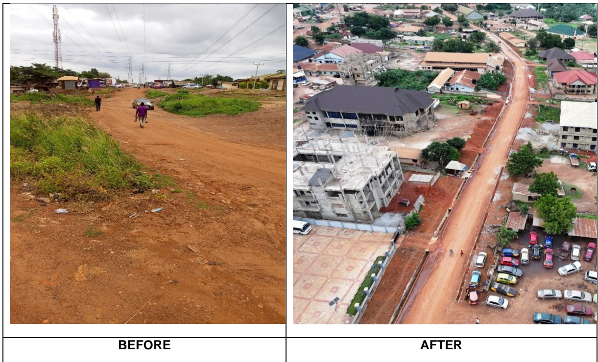
Constructed 1.40km Tarred road with 1.40km, 0.60 and 0.9m slabbed U-drain paved 1400m walkways and 47No single Armed streetlights 47No Luminaries
