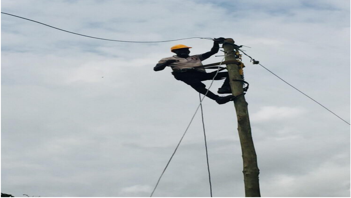
Electricity Extension- DACF-RFG
