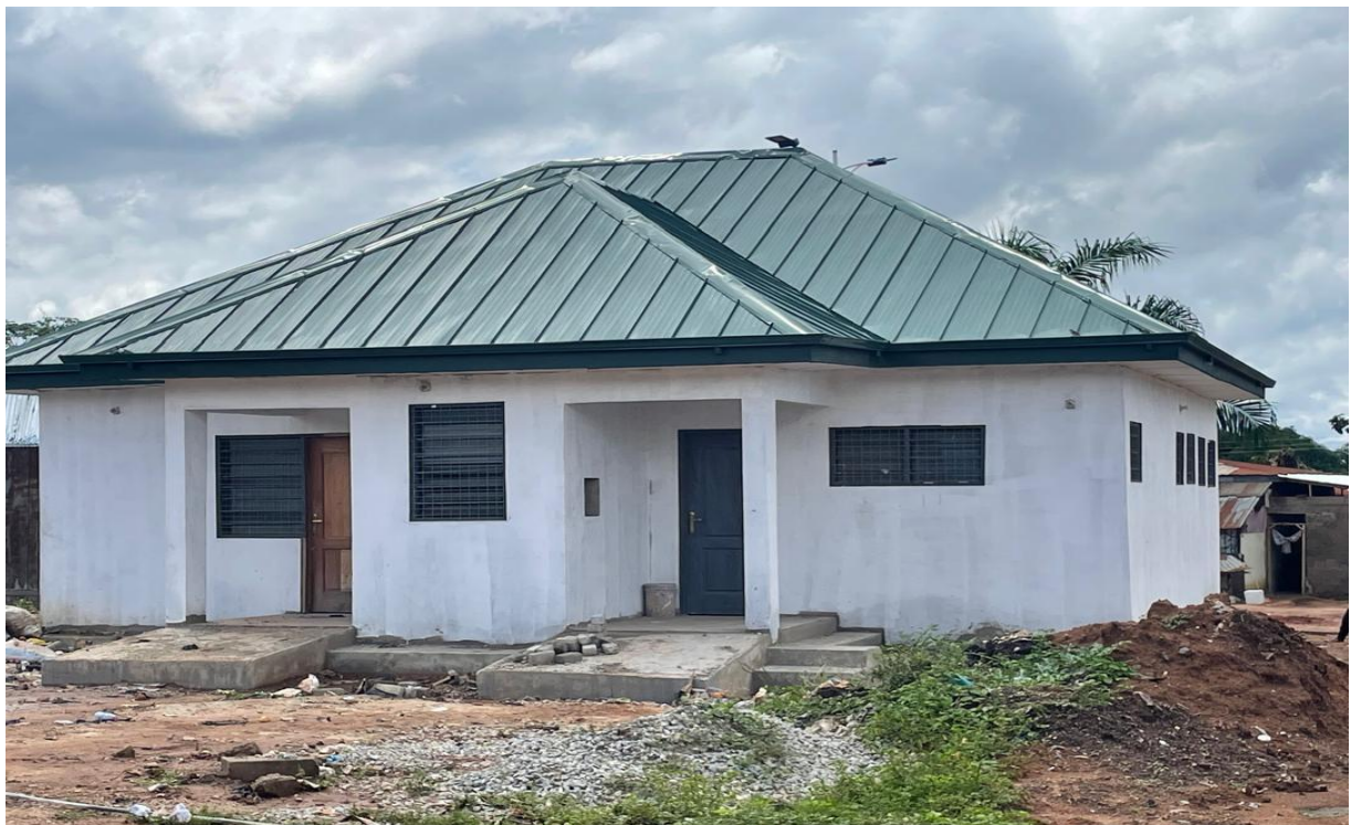
Picture 2: Construction of 1No. Sanitary Block Dormaa Ahenkro Tuesday Market (Phase-1) - (Ongoing, 90% Completed)
