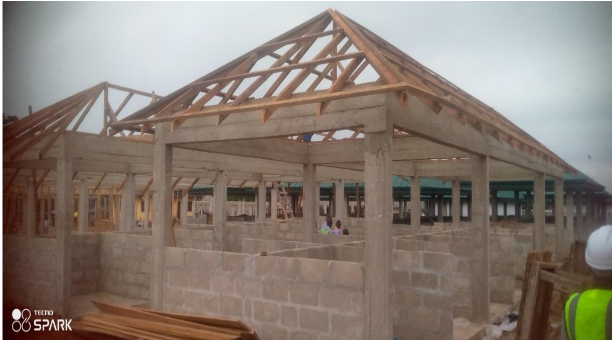
Picture 1: Construction of 9No. 14-Unit Open Market Stalls, 4No. 14-Unit Lockable Mini Stores and Paving of 2000 2 Market Spaces - (Ongoing, 55% Completed)
