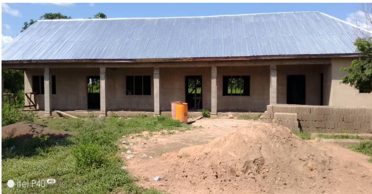
Constructed up to 66% of 1No. 3unit classroom block at Bankama Nsuoano (MP)
