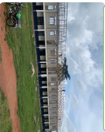
Construction of 1st Floor of 2-Storey 12-Unit Classroom Block at Wiafie Akenten SHS
