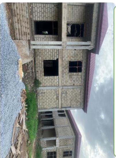
Construction of 1-NO 1-Story Classroom Block At Nkenkenu (Yaa Pokuaa Technical and Vocational Institute)
