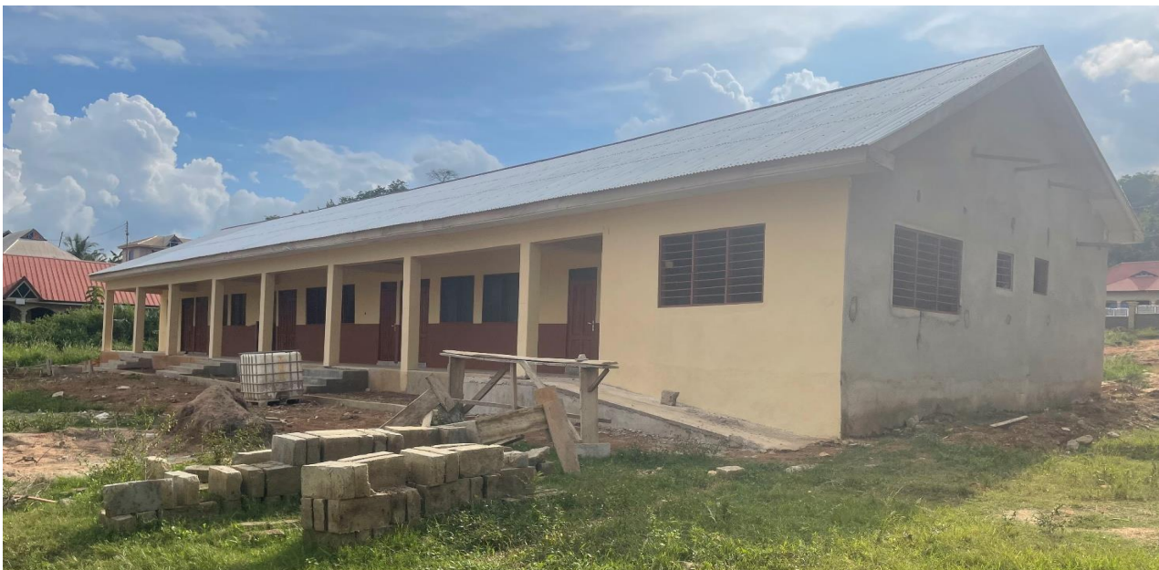
85% OF WORK COMPLETED ON THE CONSTRUCTION AND FURNISHING OF 1 NO. 3 UNIT CLASSBLOCK WITH OFFICE ,STORE , STAFF COMMON ROOM AND 4 SEATER W/C TOILET AT AHANSONYEWODEA (IGF/DACF)
