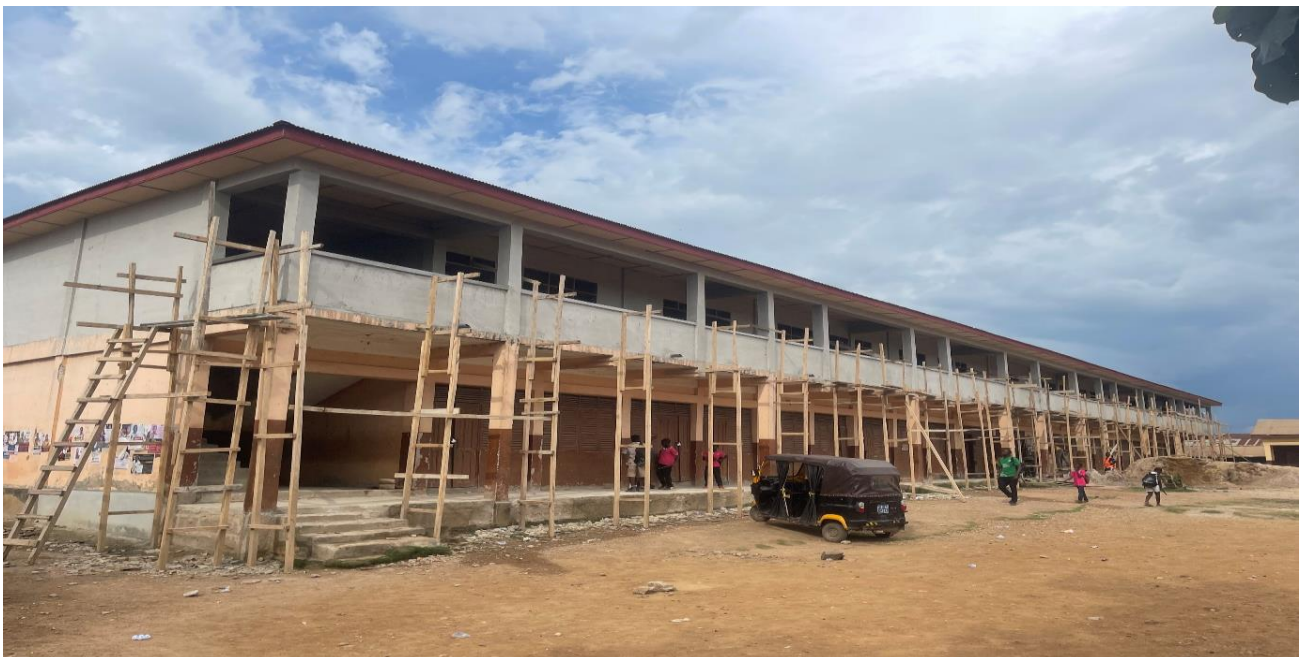
1NO. 6-UNIT FIRST FLOOR OF AN EXISTING CLASSROOM BLOCK 80% COMPLETED AT BOETE (IGF)
