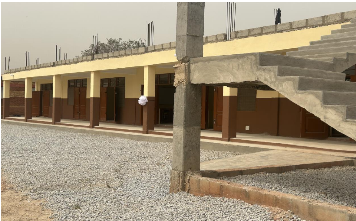
1 No. 6 -Unit Classroom Block at Adumanu M/A Primary school, phase 1 completed – DACF-RFG
