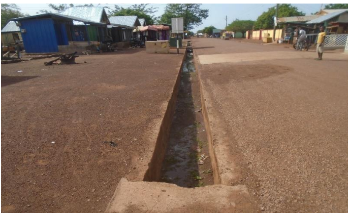
Desilting of drains along Yoo street and access road to Yoo Naa's Palace
