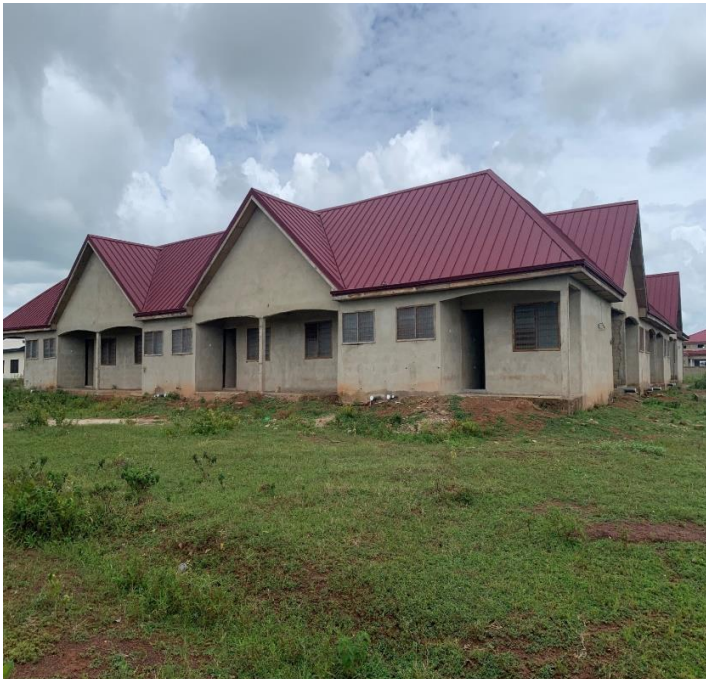
Construction of 1 No. 20 Unit Compound House for Health and GES staff at Nanton (Plastered)
