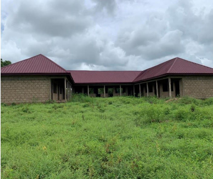
Construction of 1No. 6-Unit School Building with ancillary facilities at Zieng (Roofed)
