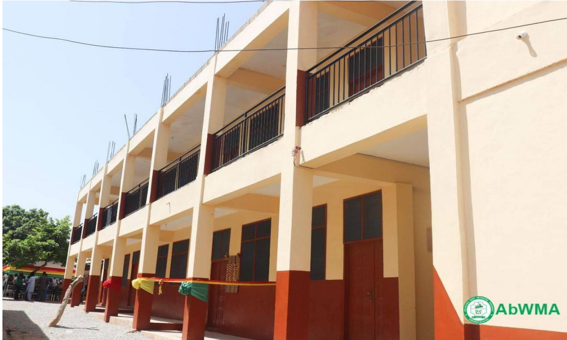
Construction of 1No. 2-Storey 6-Unit Classroom Block @ St. Augustine Ang. – 100% Completed, Handed over and In-use.
