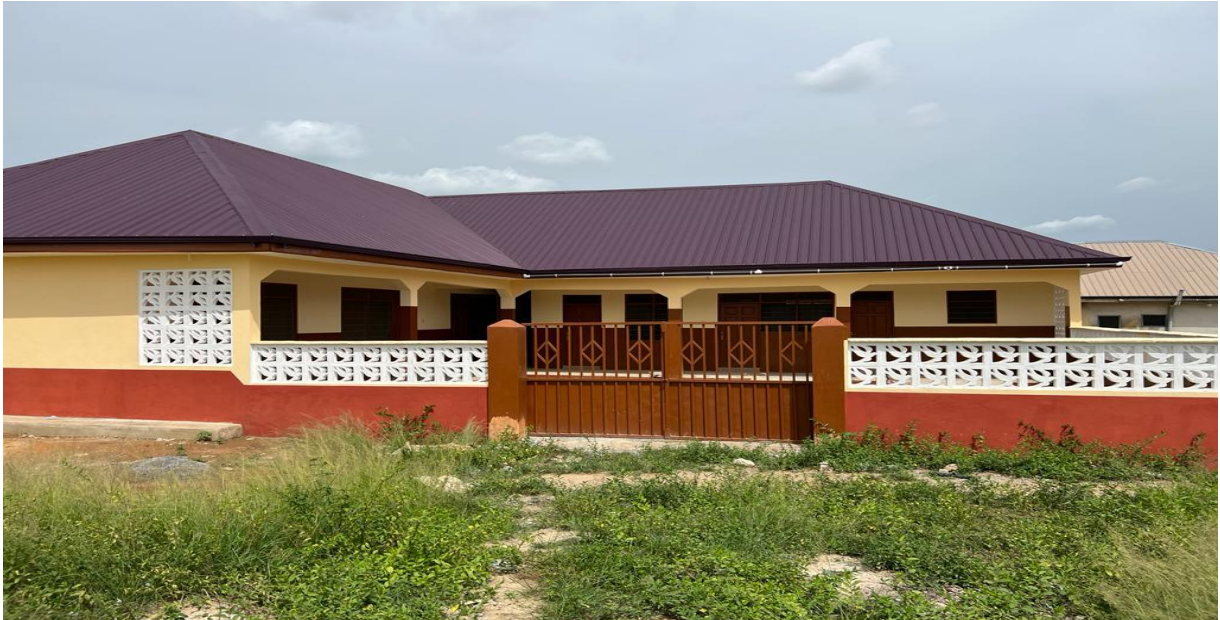
Constructed 1no. 3-unit KG block with office, store, kitchen and 4-unit W/C toilet at Saabon Zongo KG
