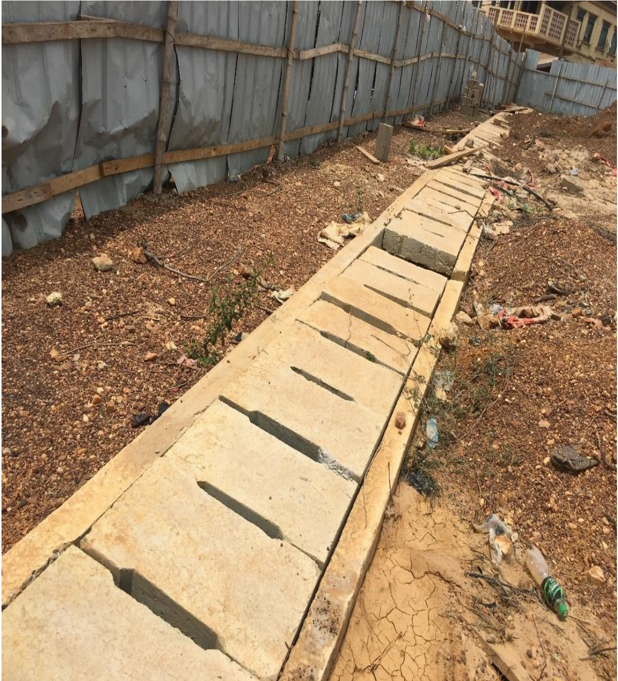
68 LOCKABLE SHOPS AT THE LINTEL STAGE OF COMPLETION, PARKED PAVING BLOCKS AND 'U' DRAIN CONSTRUCTED AT OLD PREMIER, AKIM ODA
