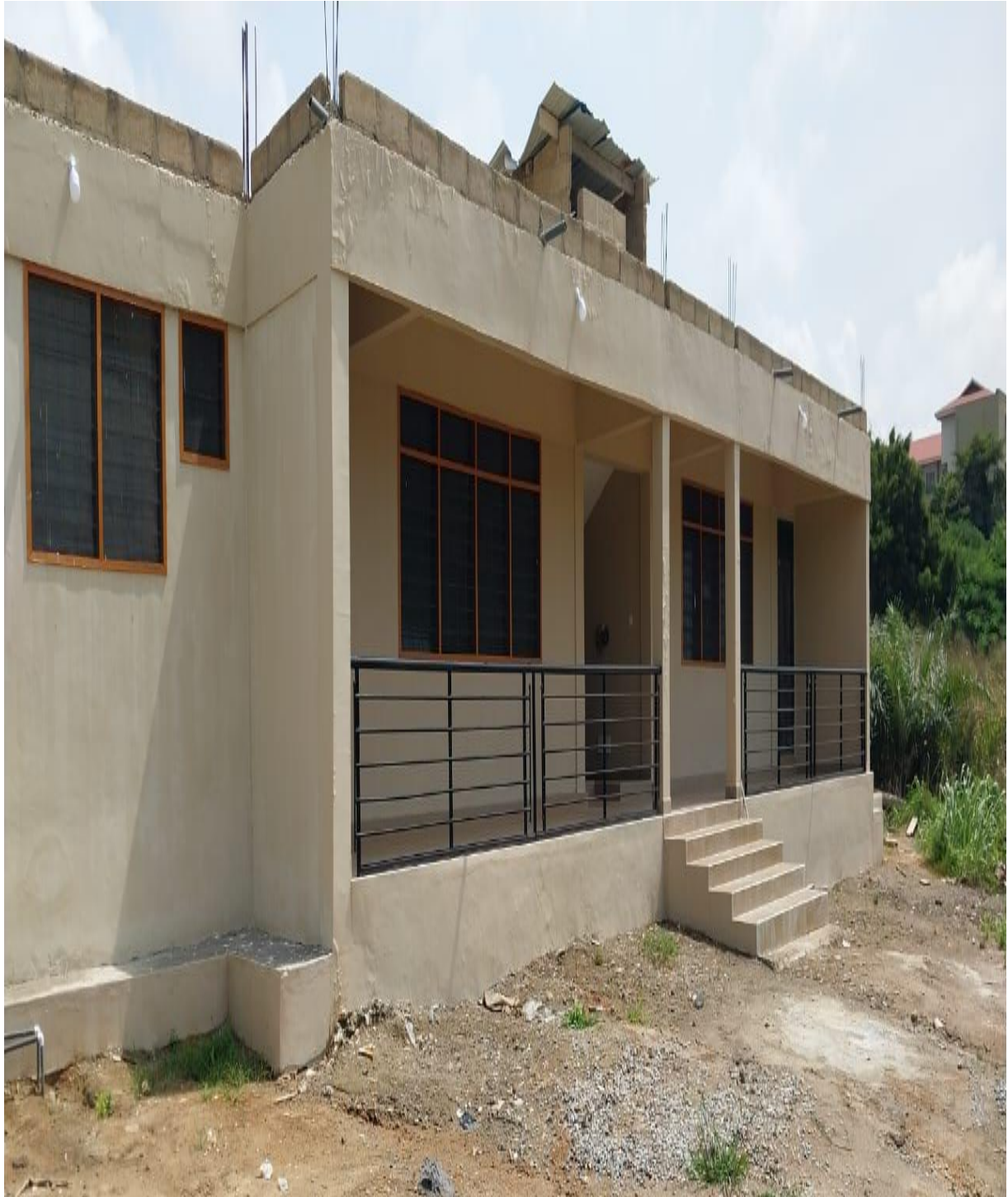
Construction of 2- unit, 2 Bedroom Semi Detached Residential Facility for Middle-Level Teachers in the Metropolis
