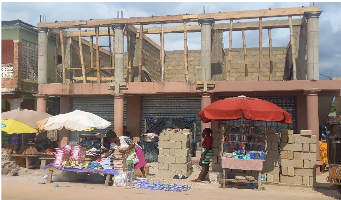
1 No. 3 Unit Trading Store at Asikuma Market Ph.II lintel level completed (Opposite GOIL) IGF
