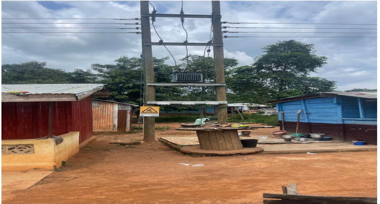
Extension of Electricity to New Communities in Duakwa.
