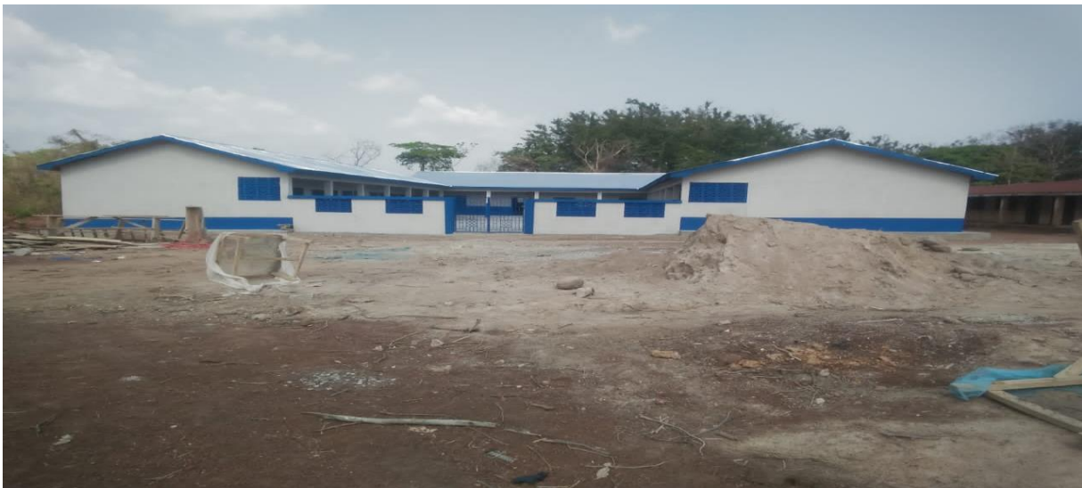
Constructed a 6-unit classroom block and staff common room at Jankufa Presby school (DACF-RFG)
