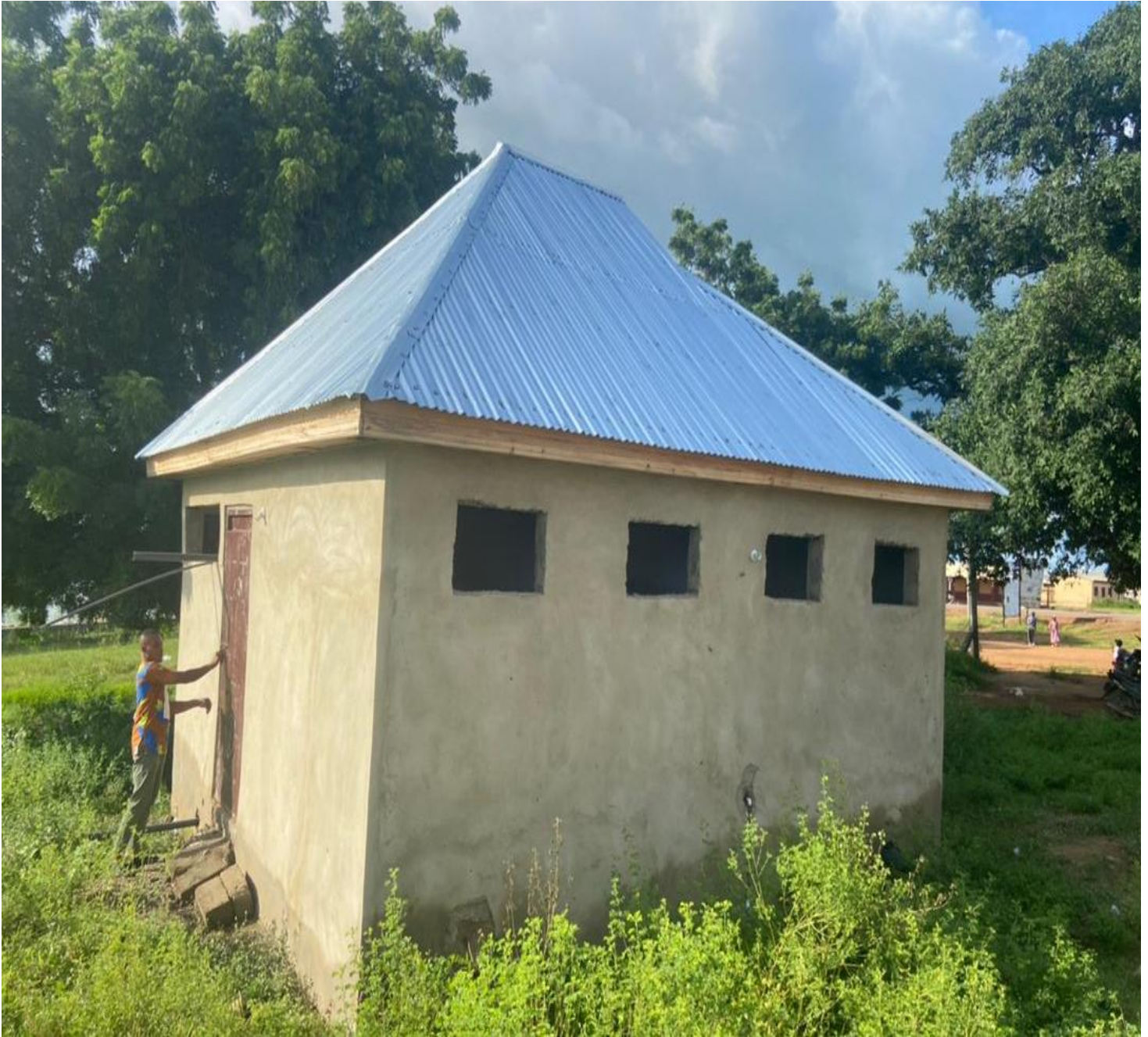
Construction of 4-seater Water closet toilet and urinals at Paga crocodile pond. Location: Paga Funding Source : IGF
