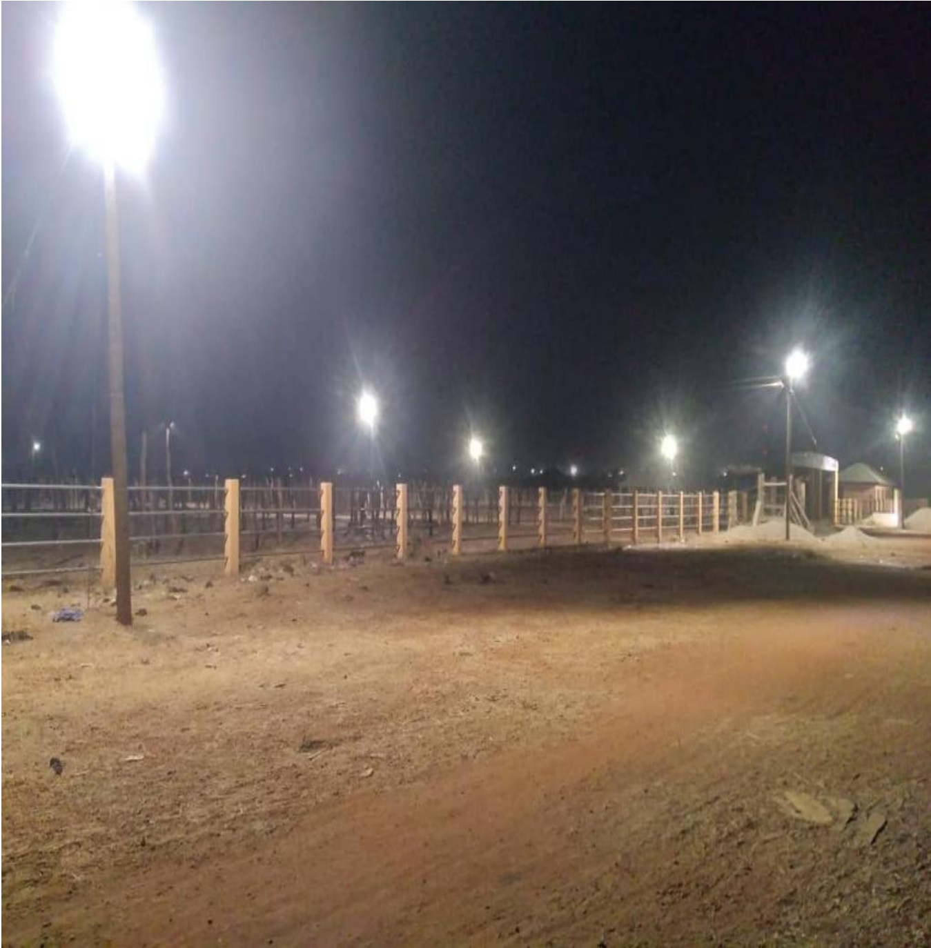
Fig. 1.3 Installed streetlight in the newly constructed cattle market
