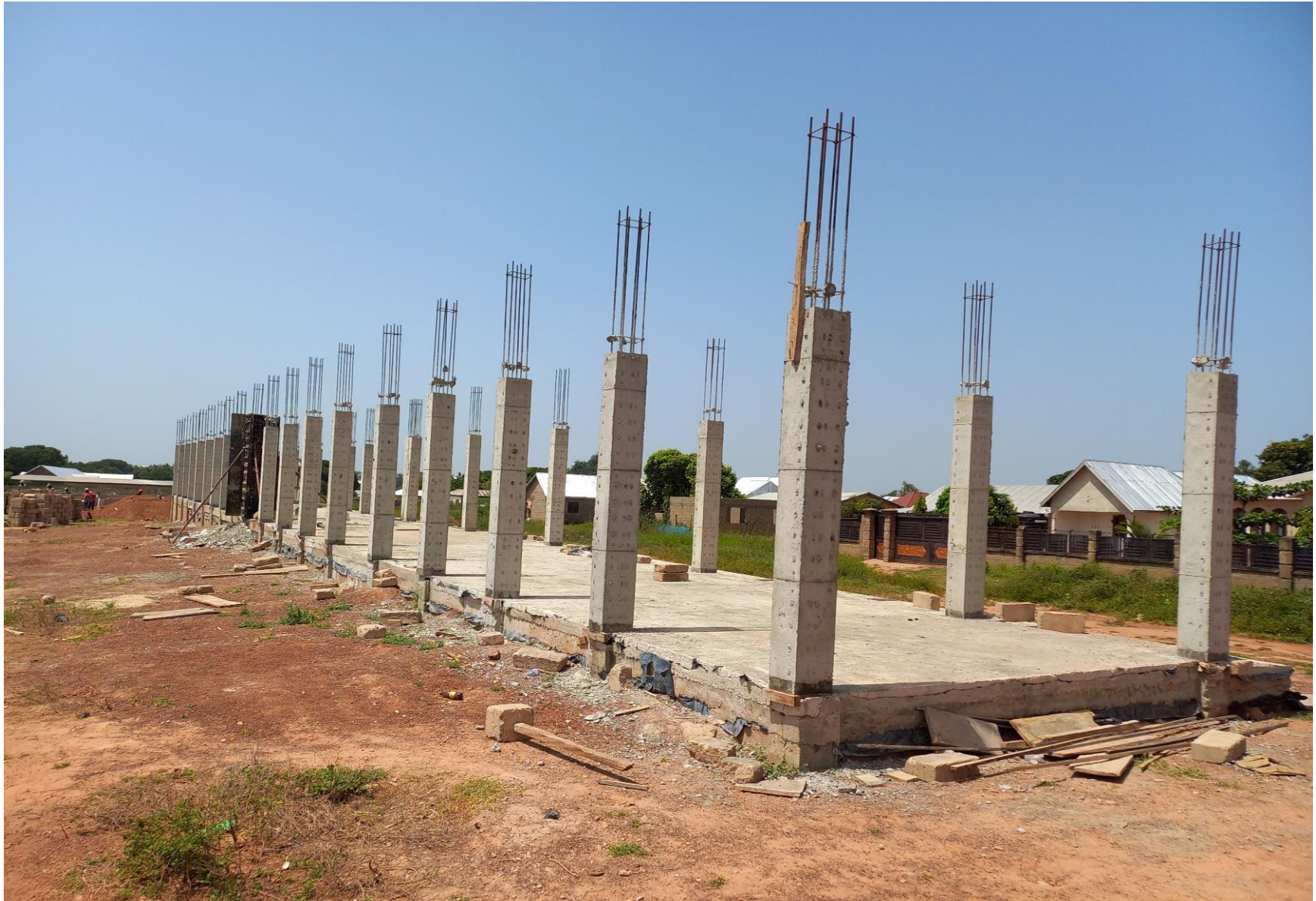
ABOVE: Construction of Commercial Building, Shed (6 No.) and External Works at Sagnarigu.
