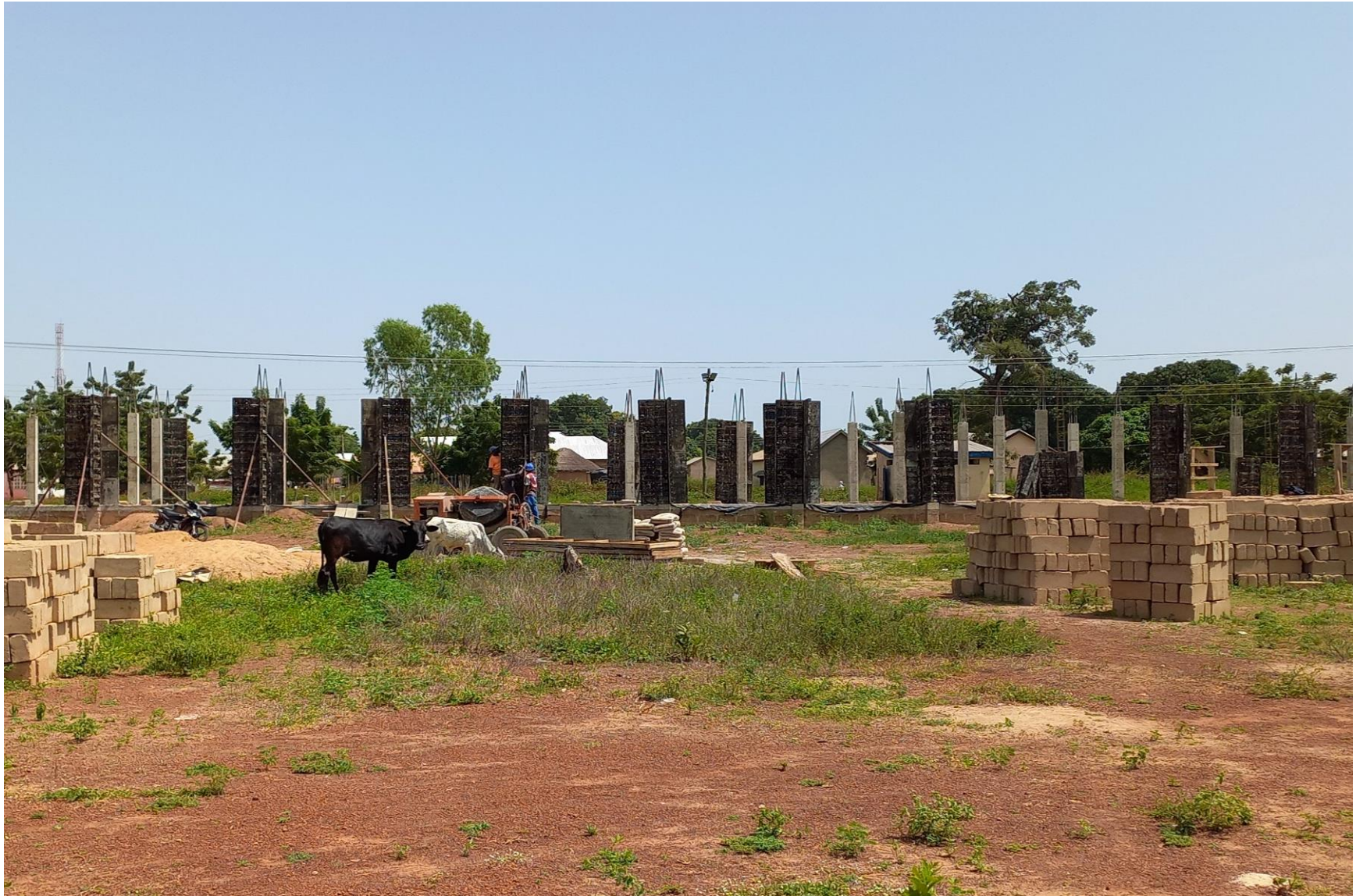
ABOVE: Construction of Clinic, crèche and construction of lockable stores at Sagnarigu.
