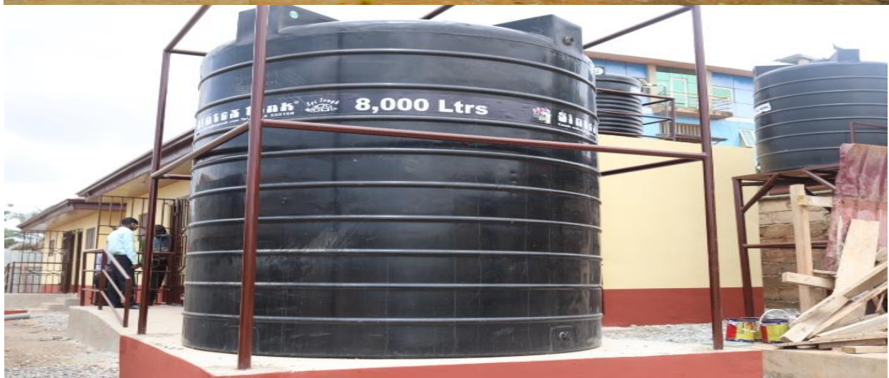
Figure 1.4 Completed 5No. Institutional Toilet with urinal, hand washing and water storage facilities at Weija, Oblogo, Joma, Gbawe and Tetegu basic schools.
