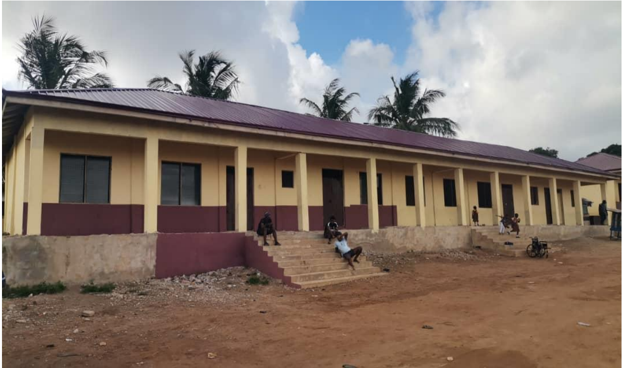
CONSTRUCTED 3 UNIT CLASSROOM BLOCK AT UNITY CLUSTER OF SCHOOLS IN MAAMOBI- GETFUND
