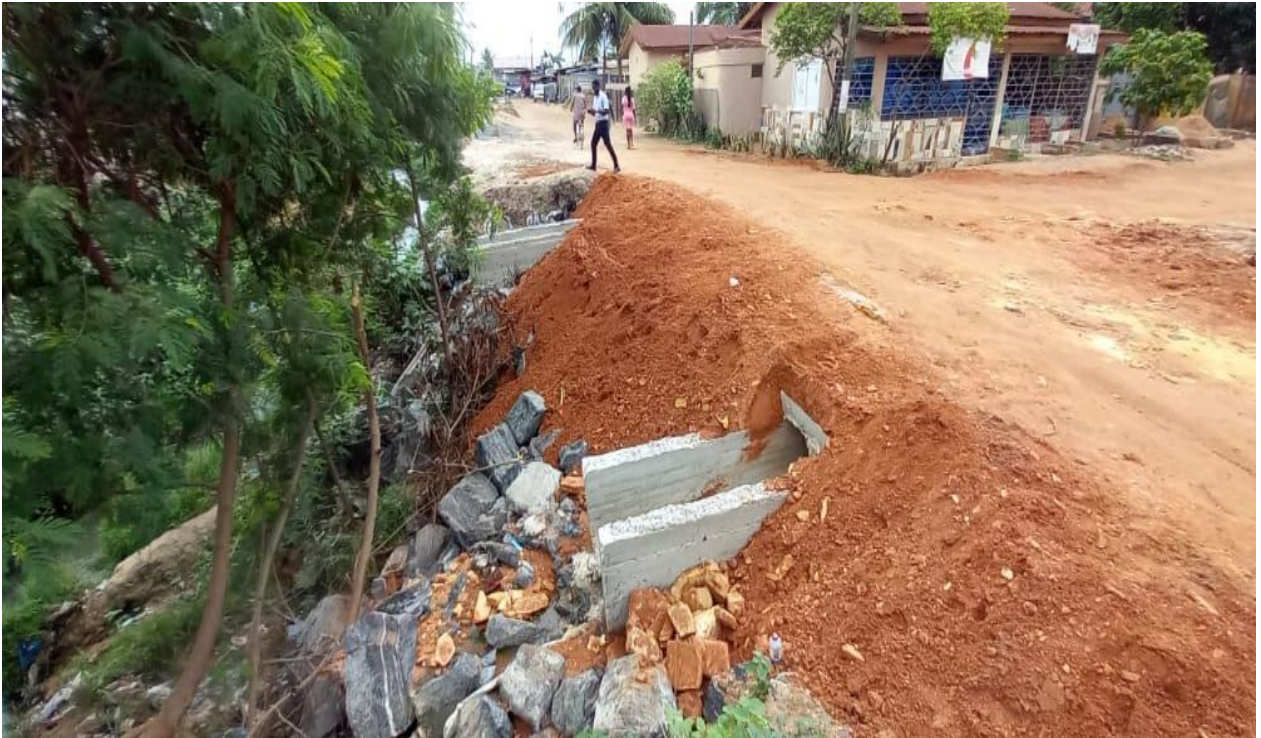
GRAVELLED WORKS AND REPAIRED DRAINS AT 3RD GATE DOWN WITHIN THE ADENTA MUNICIPALITY (NEAR OGBOJO MARKET)
