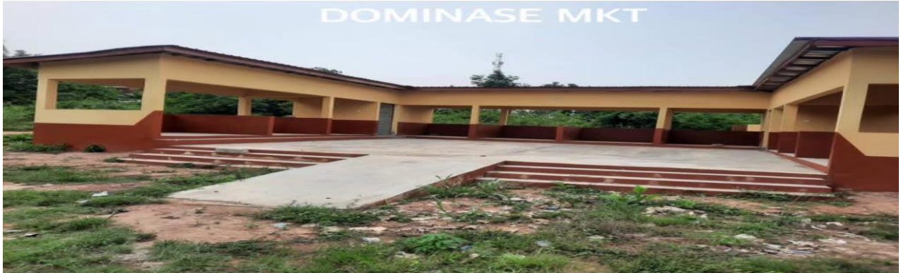
Figure 6: Completion of 1No. 12Unit Market sheds, 2No. Stores and Toilet Facility at Dominase
