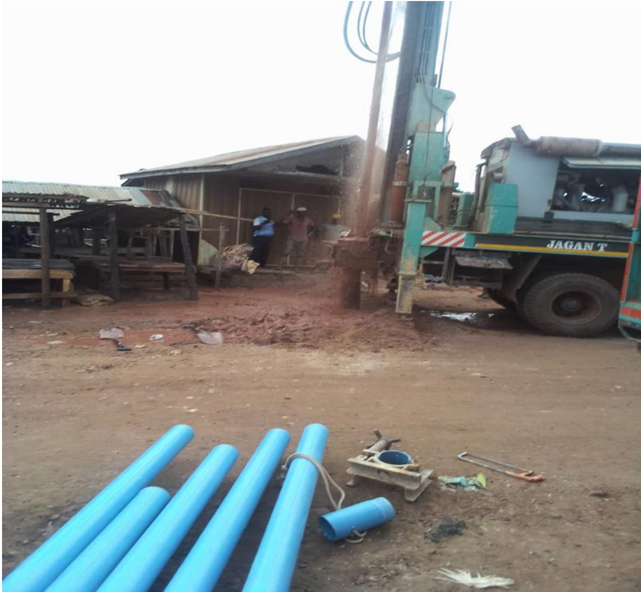
Figure 4: Drilled and constructed 2No.mechanized borehole at Wenchi maize market and slaughter house.
