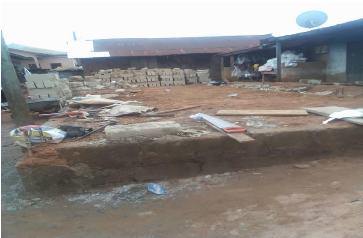
Figure 5: Constructed a washroom facility and drilled of 1No. Mechanized borehole at Wenchi old market (IGF Ongoing)
