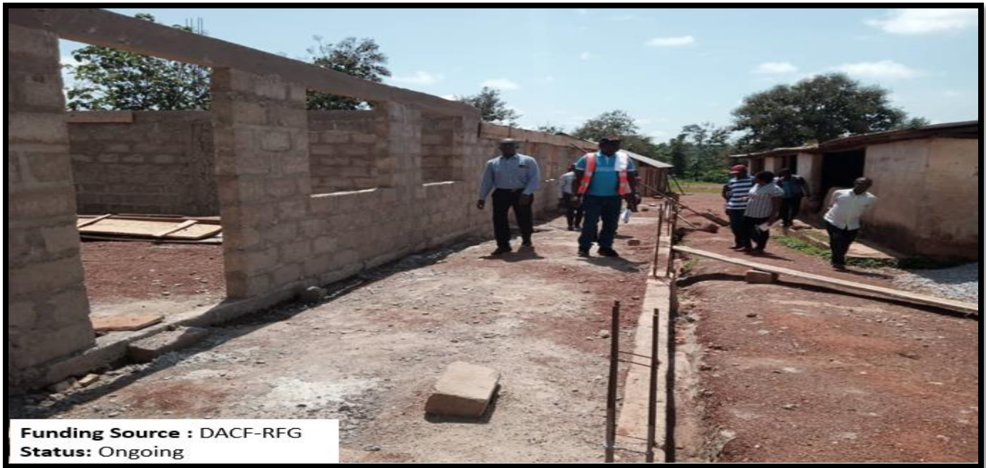
Figure 8: Construction of 1No. 3-unit classroom block for Kyeremasu SDA Primary School at Kyeremasu
