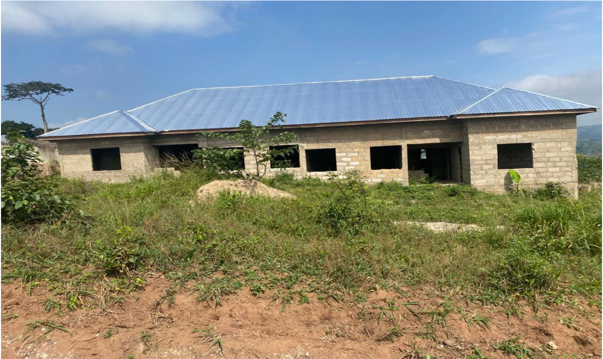
Figure 13: Construction of pavilion for fire and Ambulance service bay at Nsuta –DACF-RFG
