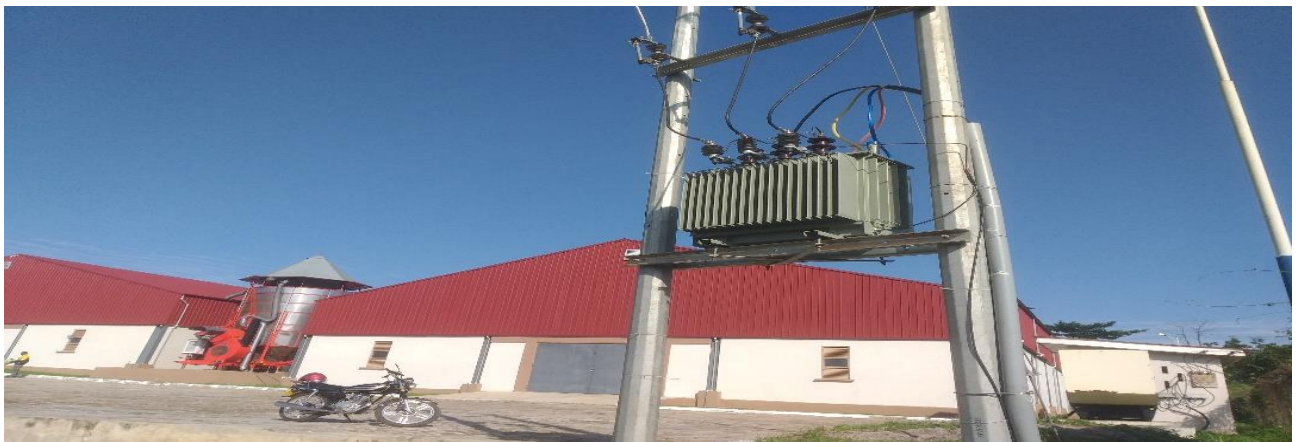
Figure 7: Procured Transformer for Maize Processing Factory (1DIF) and Connection to the National Grade –DACF
